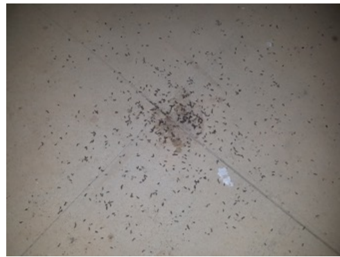
Photo 10: B1 - Concentration of bat droppings on floor of loft
