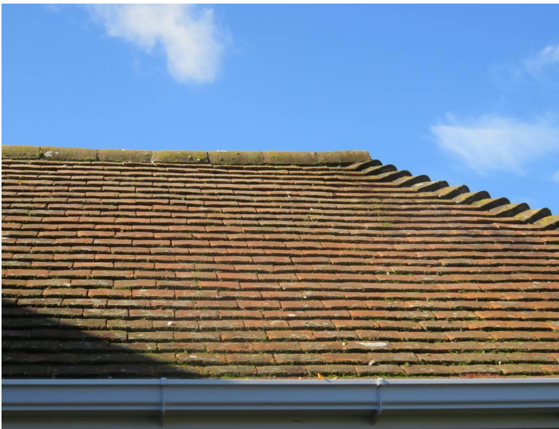
Photo 9/10 Plain tiles. These provide limited bat access potential unless damaged or lifting. Hips and Ridge tiles generally very well pointed with no access gap other than two areas of ridge and tile gaps beneath.
