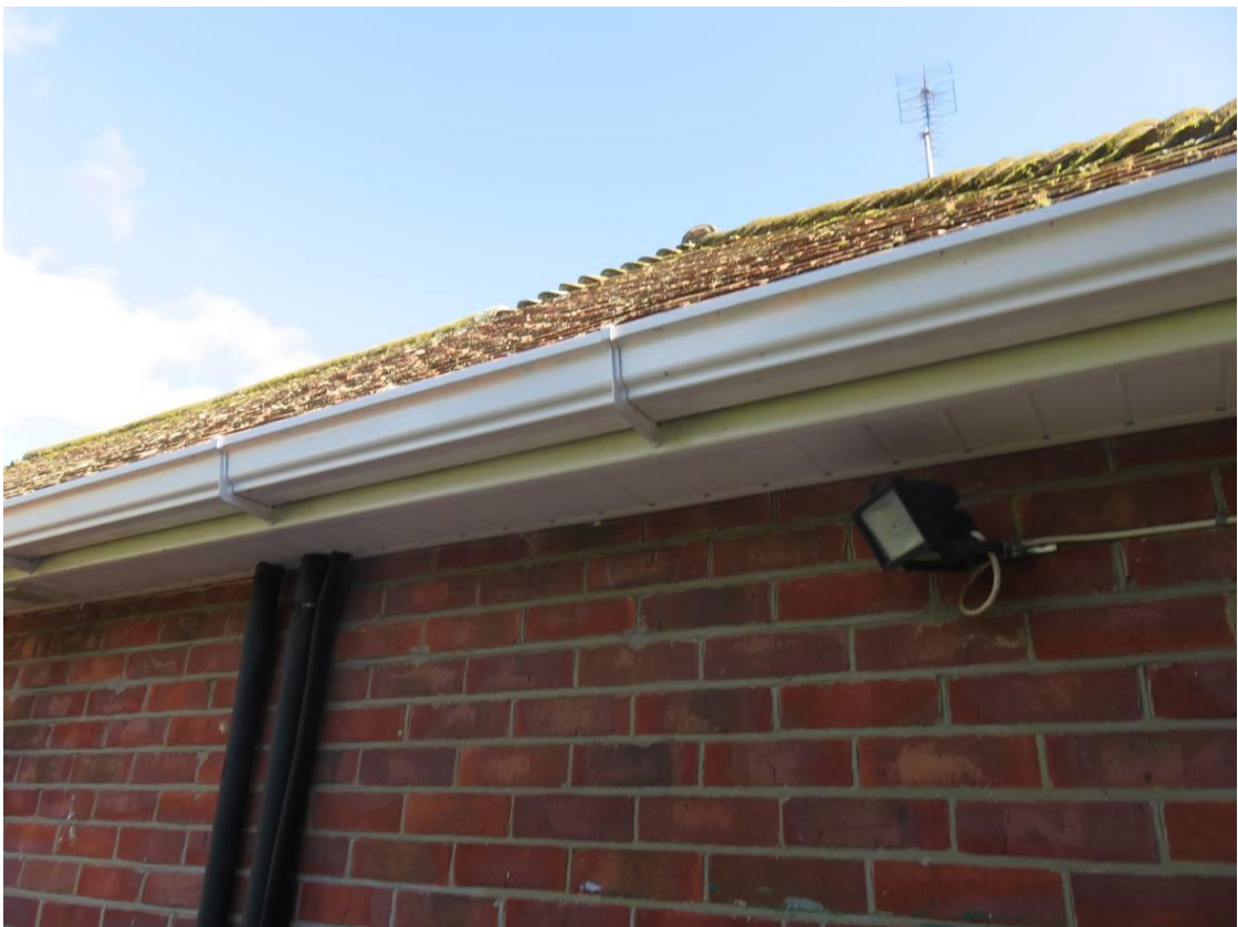
Photo 7/8 Rosebank, no potential recorded evidence or potential recorded within eaves and soffit structure
