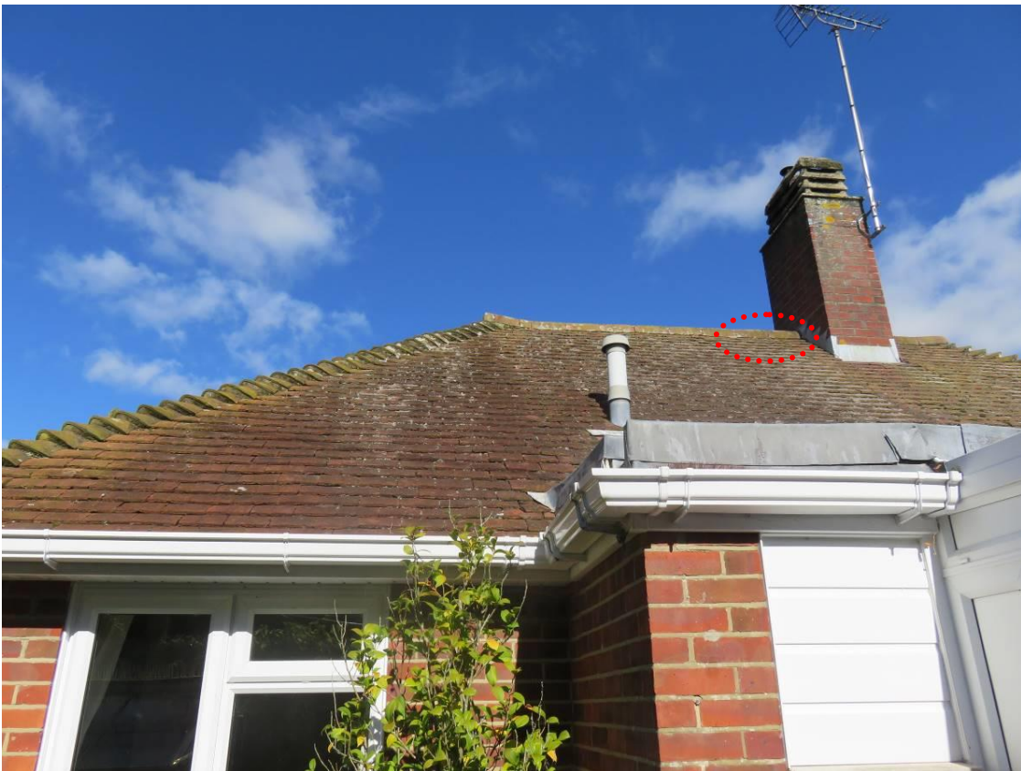
Photo 1/2 Rosebank (front North and south aspect) ridge tile gap indicated
