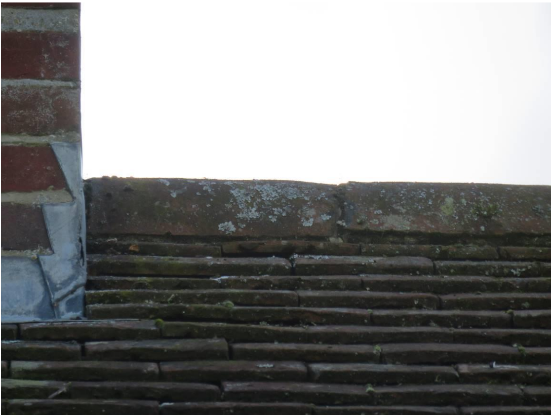
Photo 11/12 Plain tiled roof with two areas 1 north 1 south aspect by chimney with very suitable tile gap just below ridge tiles.
