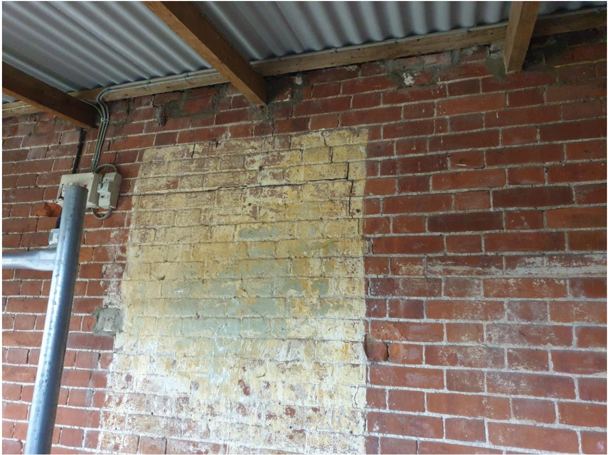
Photo 2: Internal view of cracking. Wall leans inwards above the horizontal crack.
