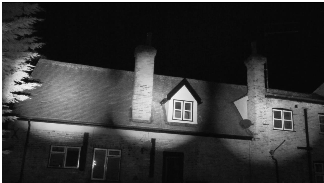
Photo 6 , screenshot from infrared camera on southeast corner angled at the east facing roof. 23 rd May 2023.
