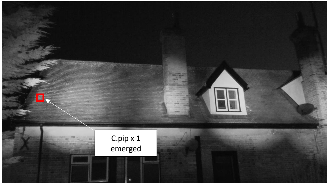
Photo 8 , screenshot from infrared camera on southeast corner angled at the east facing roof. Common pipistrelle roost beneath lifted tile highlighted in red. 22 nd June 2023.
