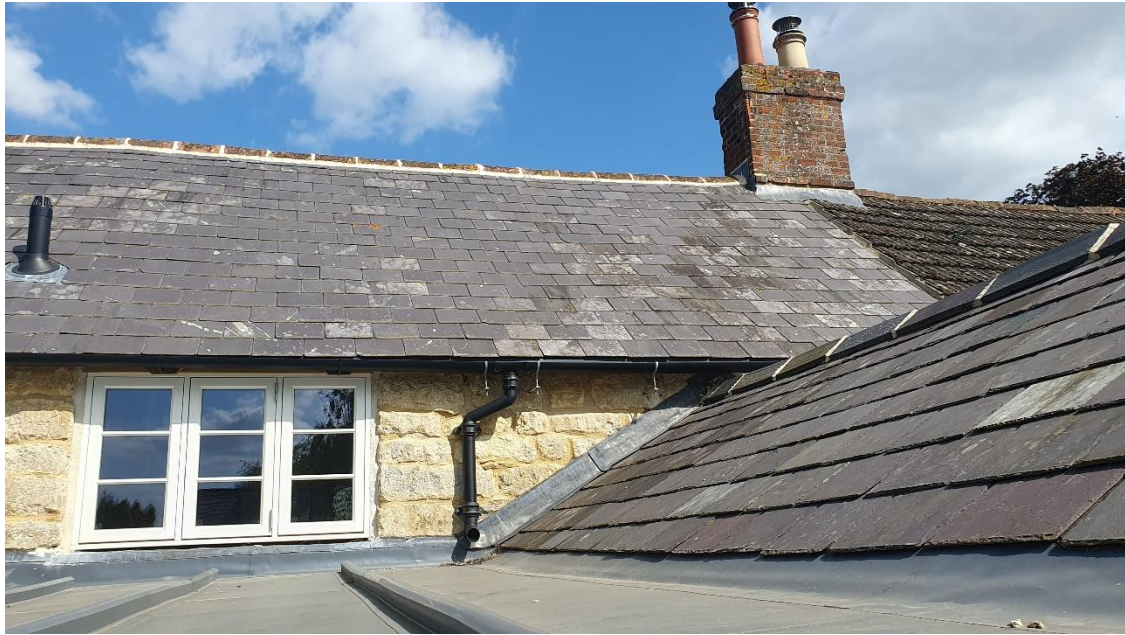
Image 5 – Final slate roof installation completed for No 3-4. This slate will continue to the right, as part of replacing the clay pantile roof tiles of No 1-2.
