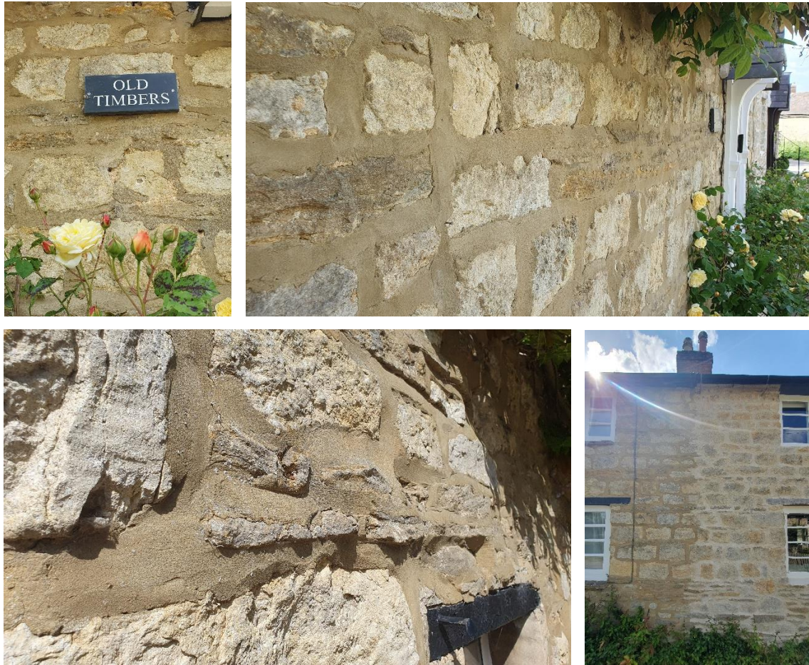
Image 6 – Photos showing the condition of the existing mortar, which is to be raked out and replaced with a new lime mortar.
