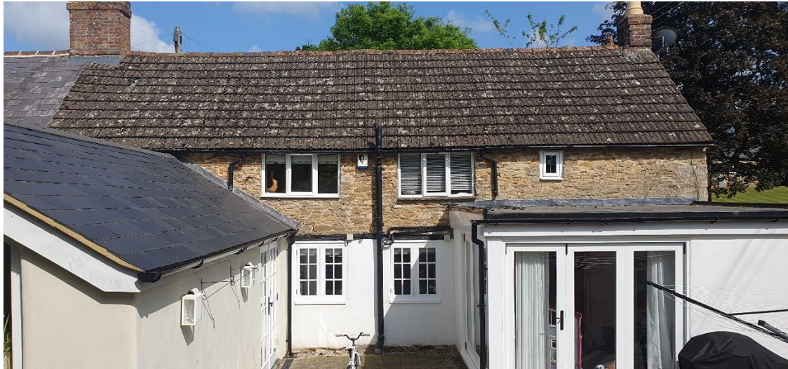
Image 3 – Photo showing the rear (West) elevation of No 1-2. Existing clay pantile roof to be removed and replaced with reclaimed purple Welsh slate to match that installed on No 3-4.
