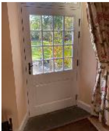
New front entrance door to extension to match existing timber glazed panelled door to the south entrance of the main house.
