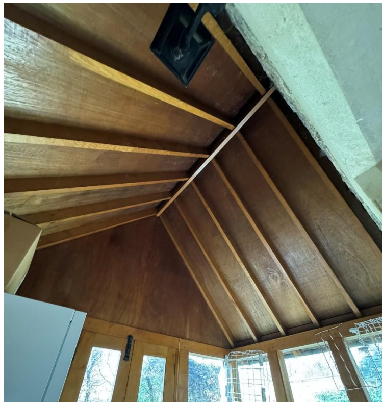
Fig.18 Internal View of Porch roof structure. Insulation to be installed between rafters and lined with plasterboard and skim
