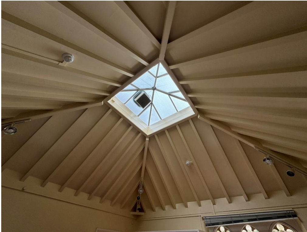
Fig.15 Existing roof structure. Insulation to be installed between rafters and lined with plasterboard and skim. Lantern to be replaced.
