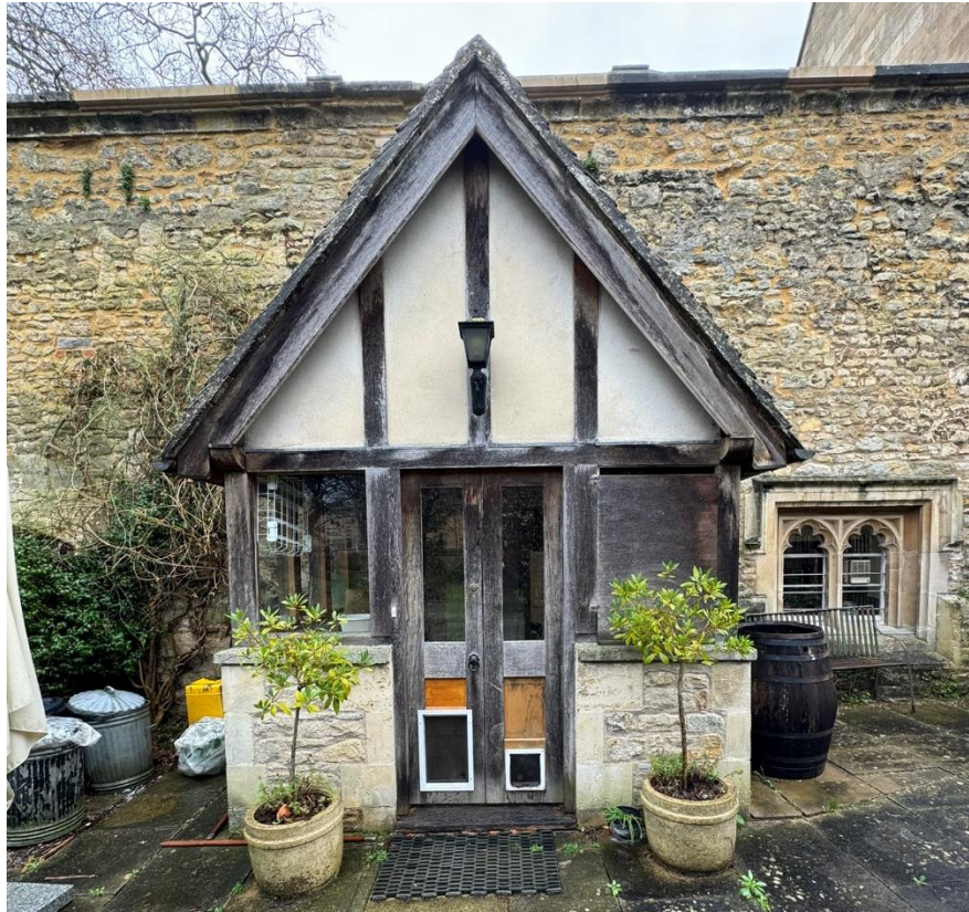
Fig.7 North East External Elevation of Existing Porch. Replacement doors proposed to match existing style. .
