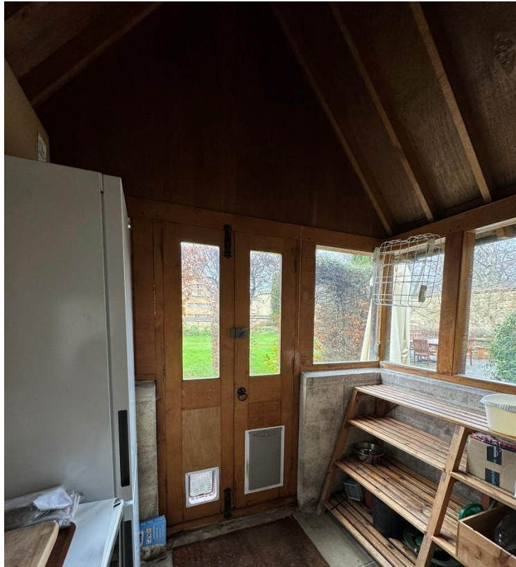
Fig.17 Internal View of Porch. Door to be replaced to match existing.
