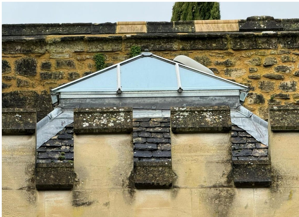
Fig.8 Existing Rooflight to be replaced with patent glazing system to match style of existing with lead covers to hips.
