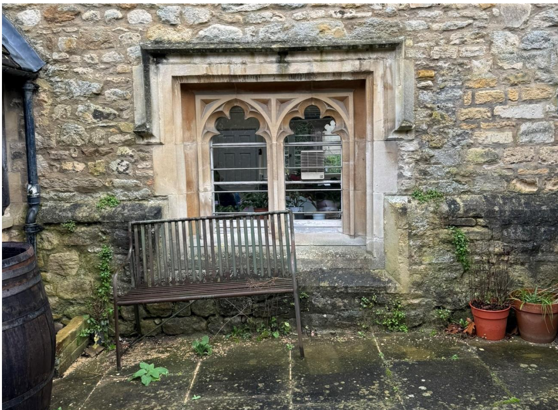
Fig.6 Existing 2-Light window to North East Elevation. Replacement window proposed to match existing.
