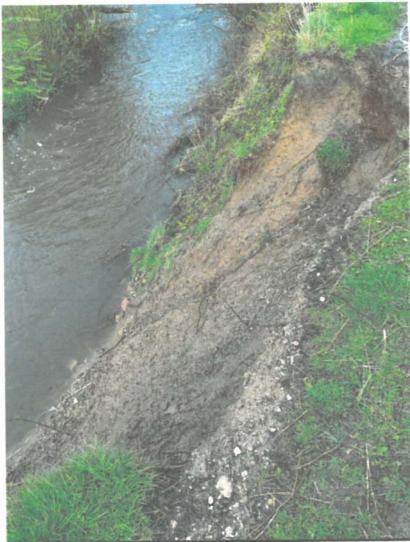
Photos of the steep banking which is the closest point of the River Wyre to the site (Myerscough football pitches seen in the background). Due to the River's narrowness during peak flow events it is fast flow and does not rise up the banking.
