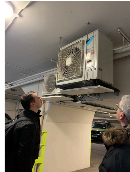
Left: Area for the air-source heat pumps
