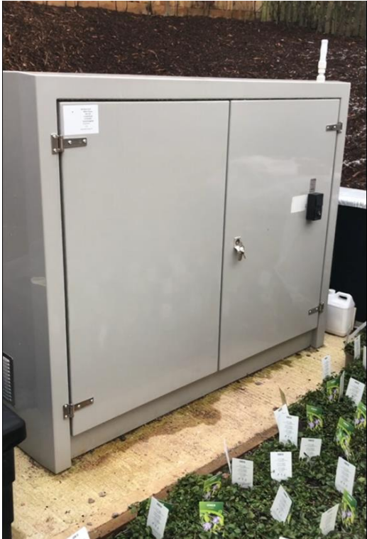
Figure 3.3: Swimming pool heating system enclosure (as installed)
