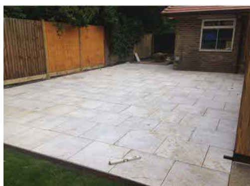
Photographs showing the snooker room and patio where the jacuzzi, sauna and games have been constructed (dated August 2014)
