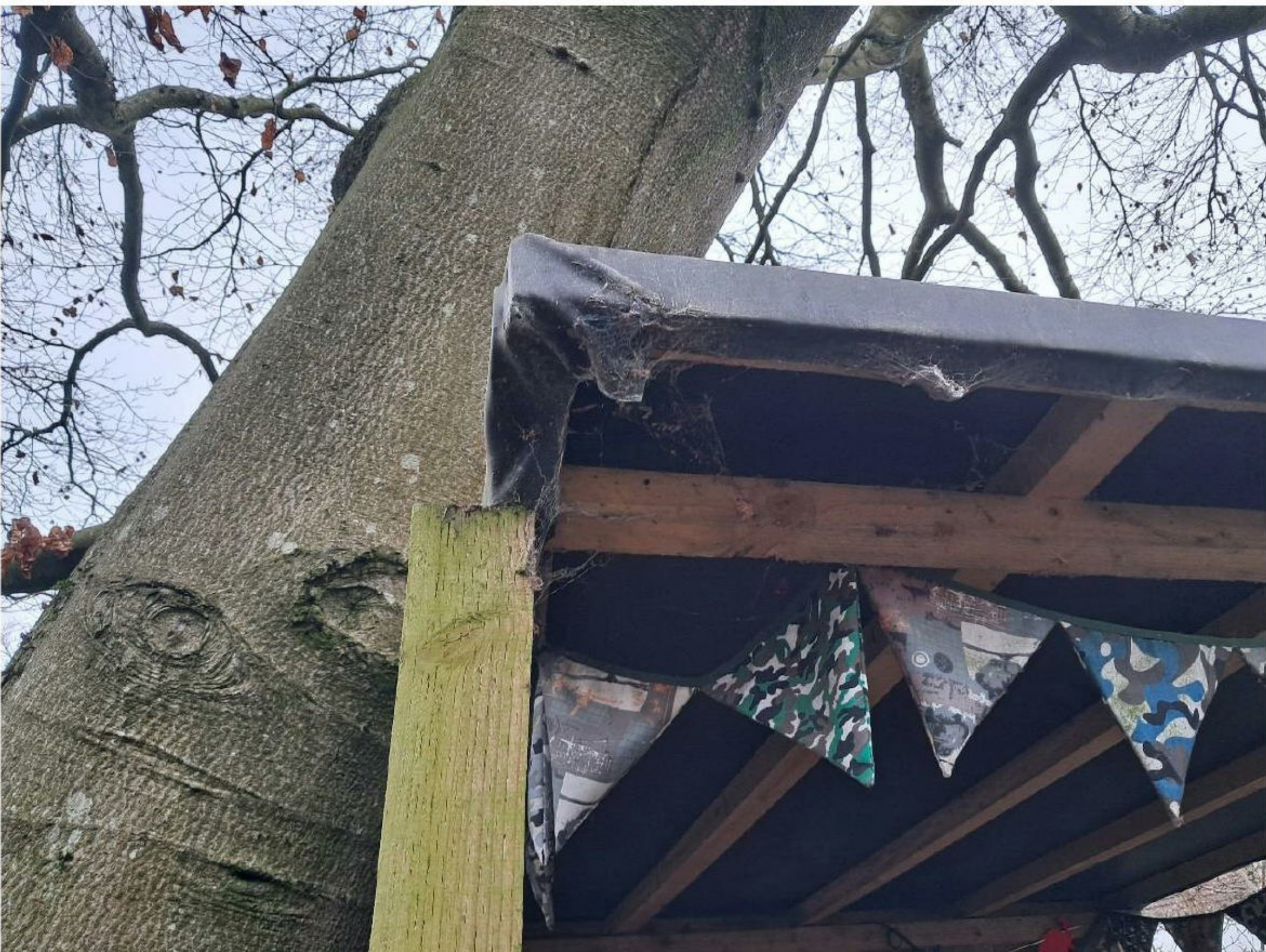
Photo 5 – Shifted roof of children's play fort.
