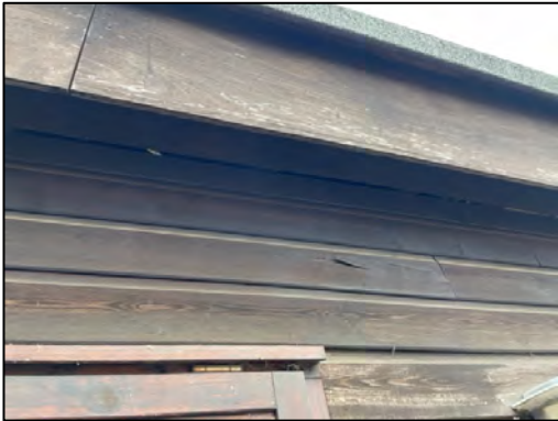
Photograph 13: The gap where the soffit box does not meet the wall on the northern elevation of building B8.
