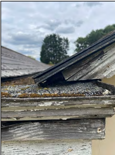
Photograph 7: The damage on the southern gable end of building B9 which could provide potential bat roosting opportunities.
