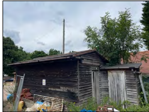
Photograph 14: The south-eastern elevation of building B3. Photograph showing the damaged weatherboarding on this elevation.
