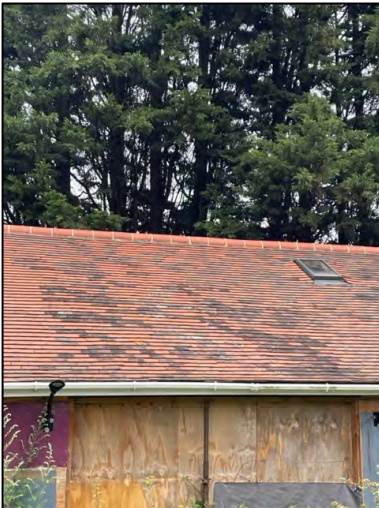
Photograph 3: The lifted tiles on building B2.
