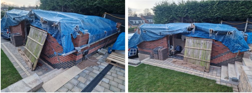
Figure 5 Current Situation demonstrating the land has been dug down to provide a level concrete plinth for the building to sit on.
