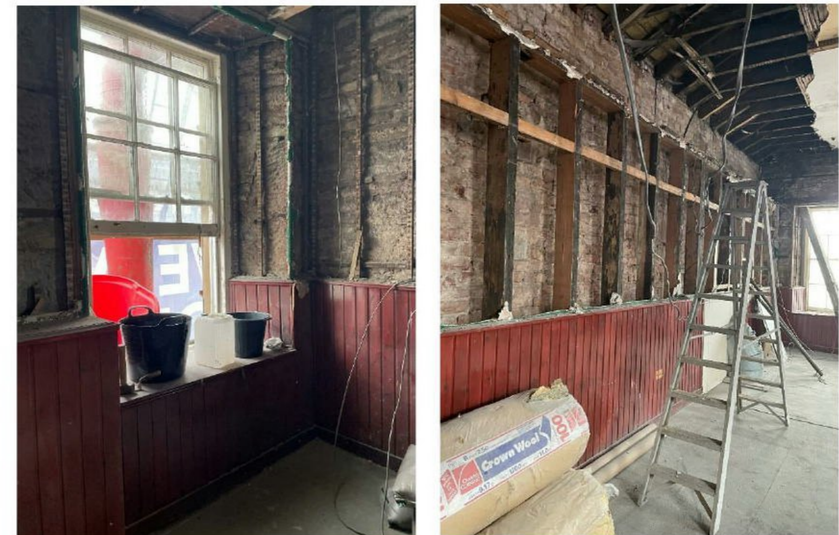
Photographs of the first floor void which is to be the staff facilities
