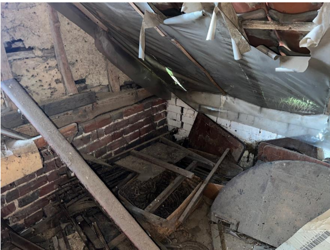
Photo 37. Shows south-west corner of loft space. Shows crack in wall. Gap between horizontal timber and brick work and light ingress.
