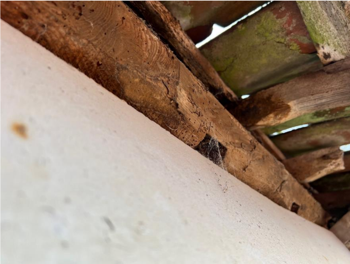
Photo 24. Shows mortice gaps under eaves along front of barn.
