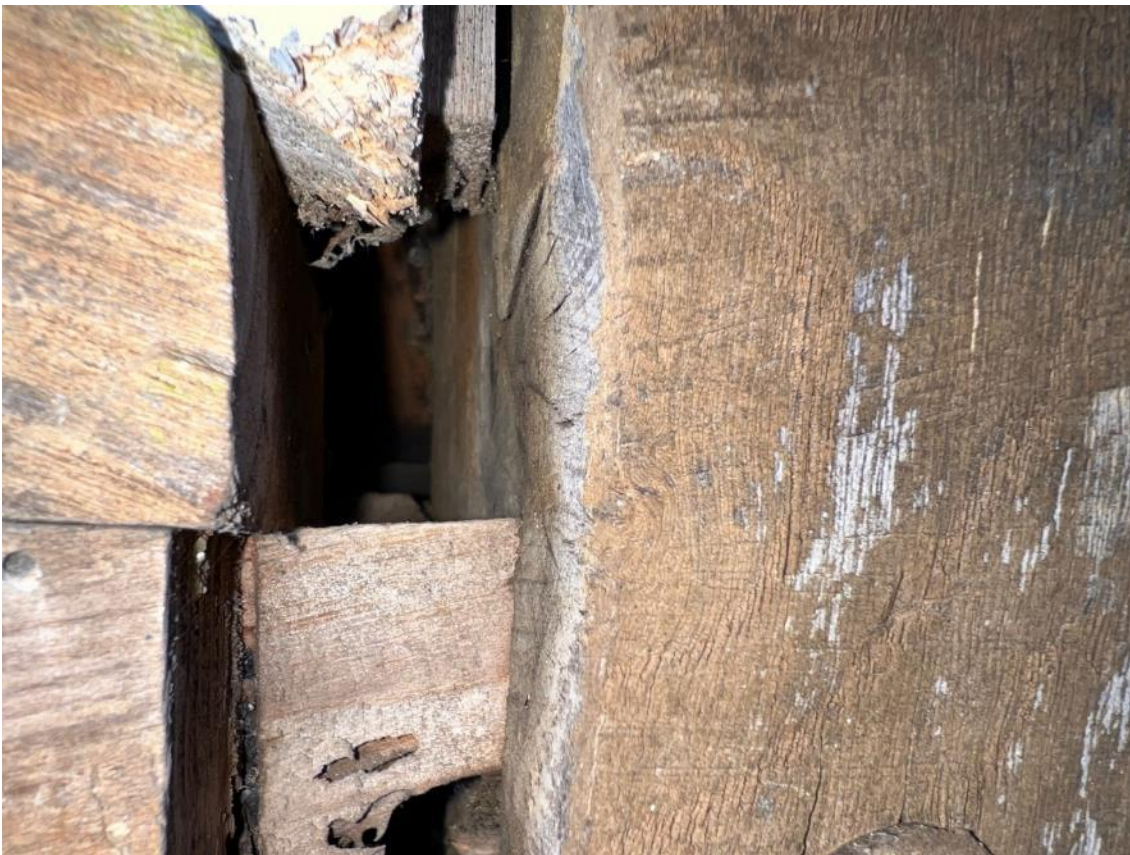
Photo 23. Close up of void as shown in photo 22.
