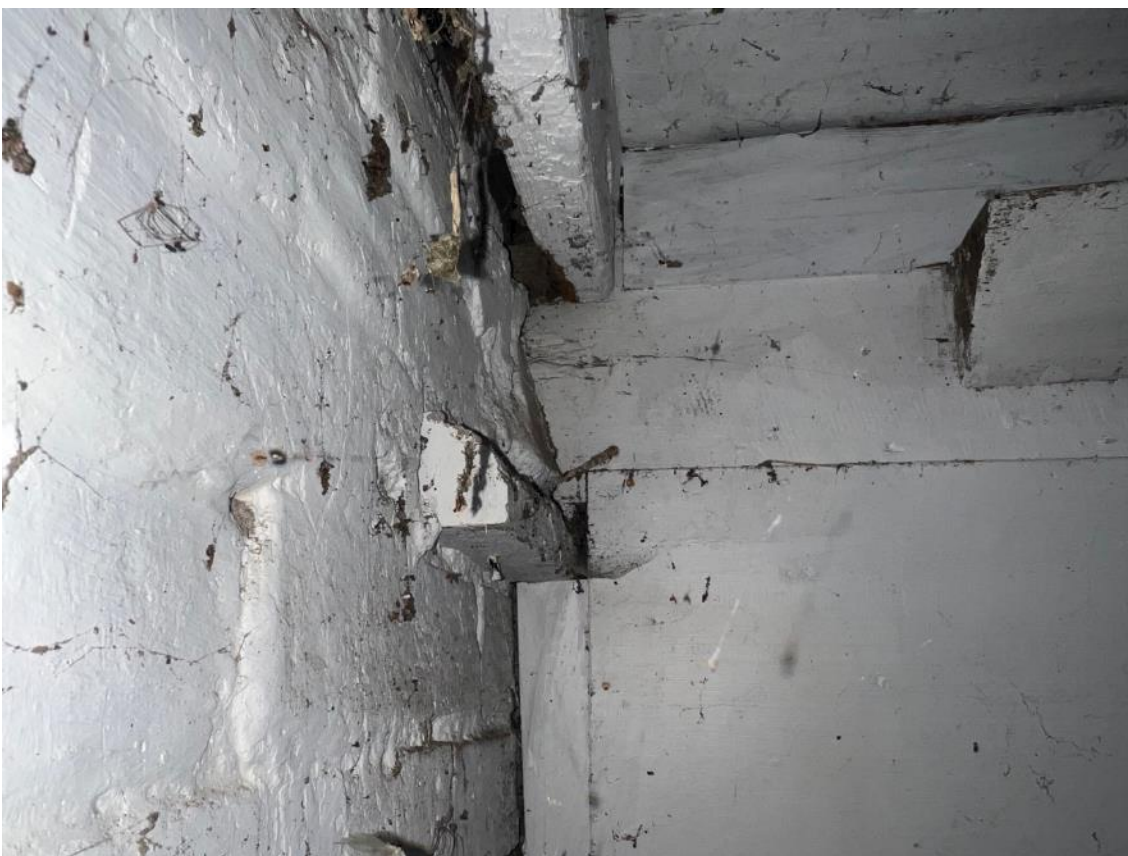
Photo 14. Shows gaps between timber and brickwork. B1.
