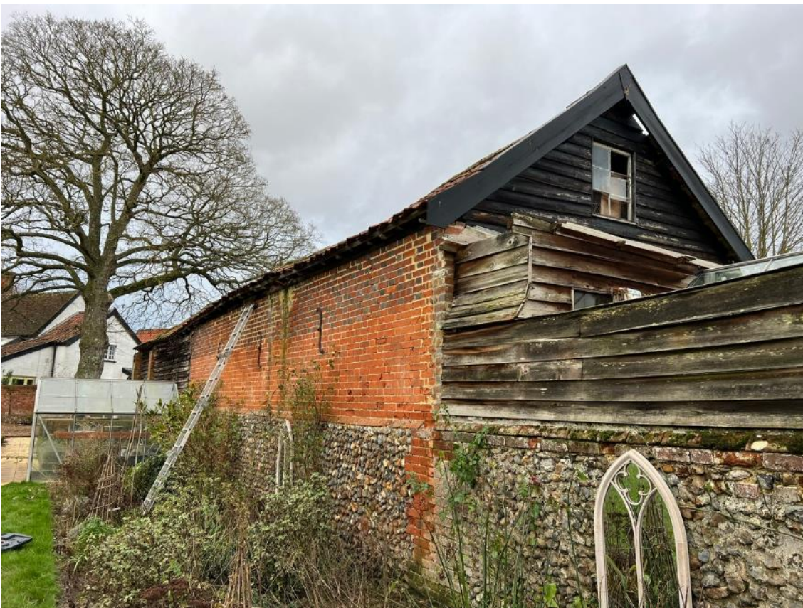
Photo 6. South-west corner of barn. Shows brick wall heading south of barn. Close up of ornamental shrubs.
