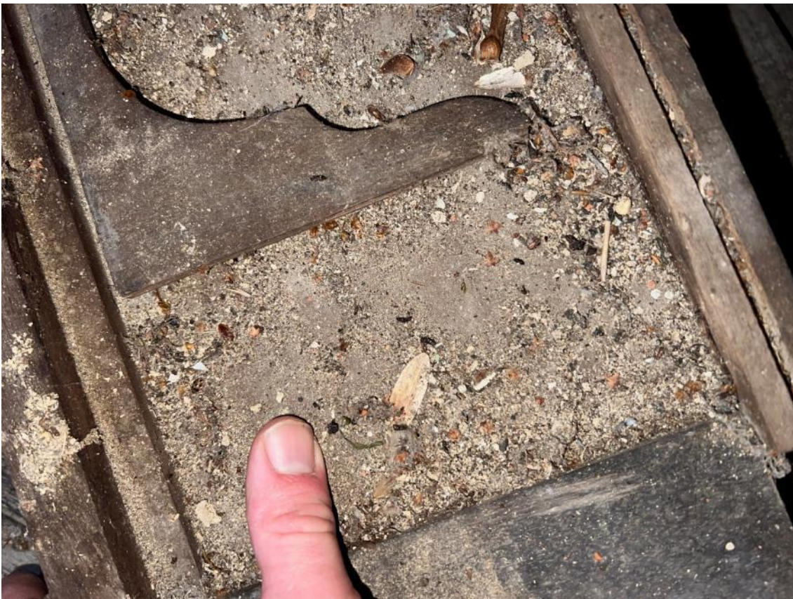
Photo 39. Shows butterfly wings, and mice droppings. South end of barn.
