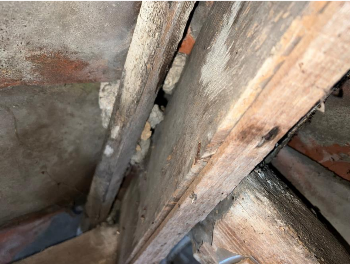
Photo 40. Shows gap between ridge board and purlins.
