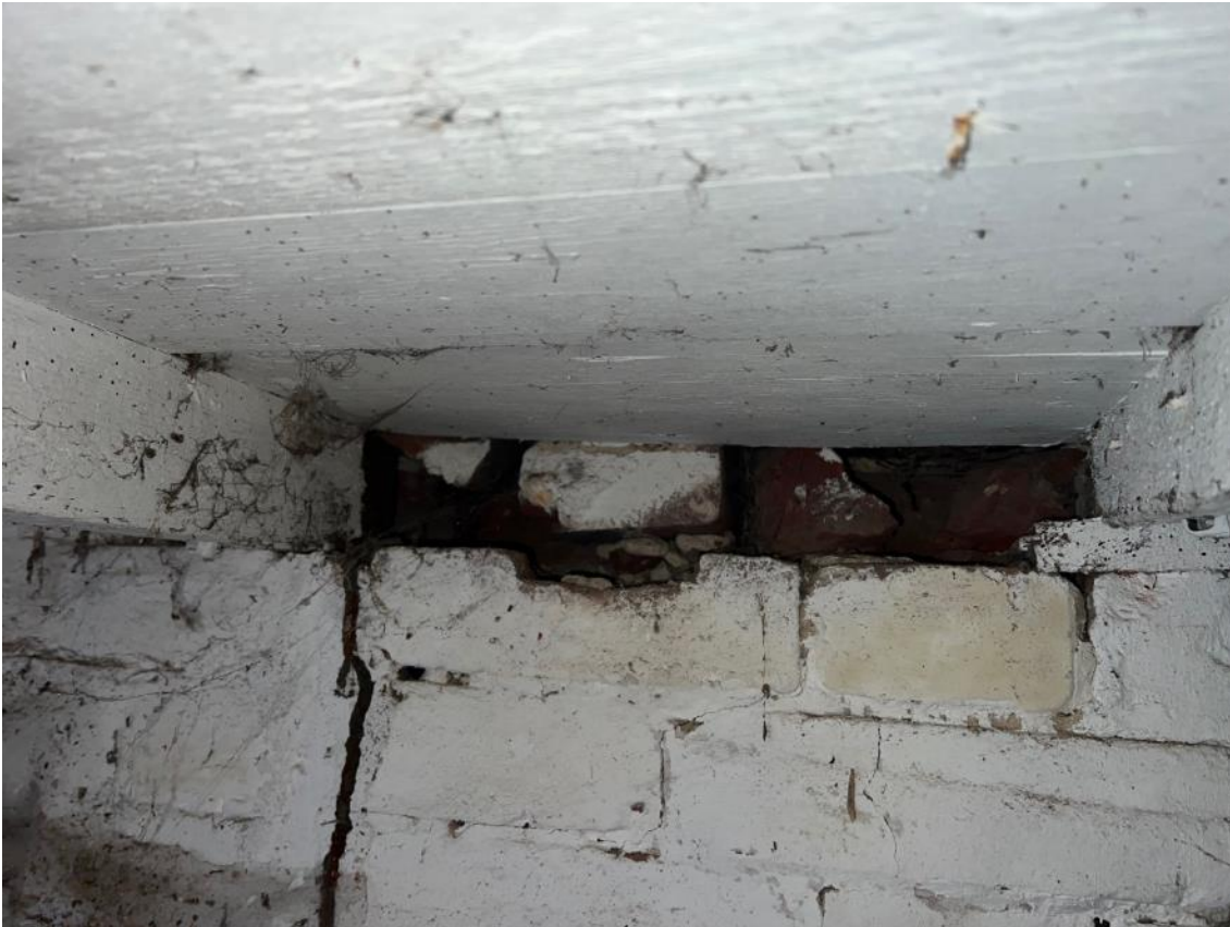
Photo 15. Shows gaps between ceiling joists and brickwork. B1.
