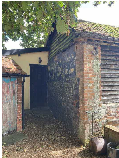
Fig 5 – North-West Elevation – Rear gable end of existing outbuilding, viewed from neighbouring garden.
