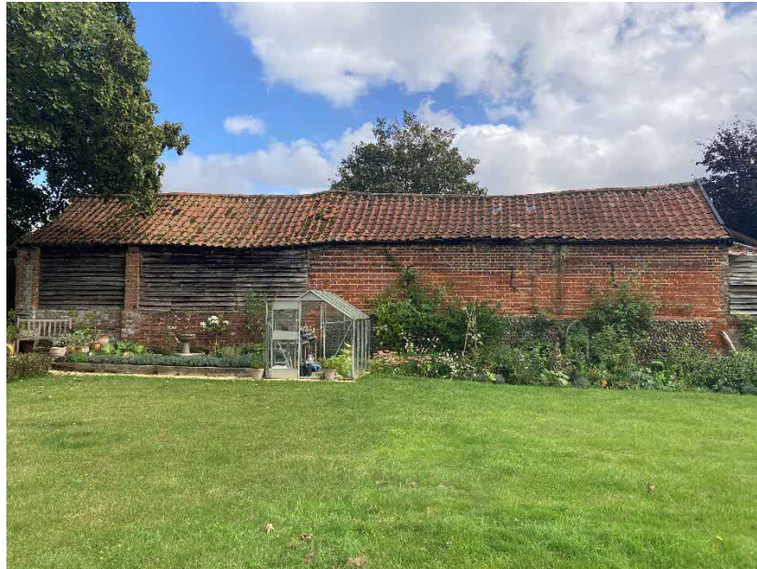
Fig 1 – South-West Elevation – Rear side elevation of existing outbuilding, viewed from neighbouring garden.
