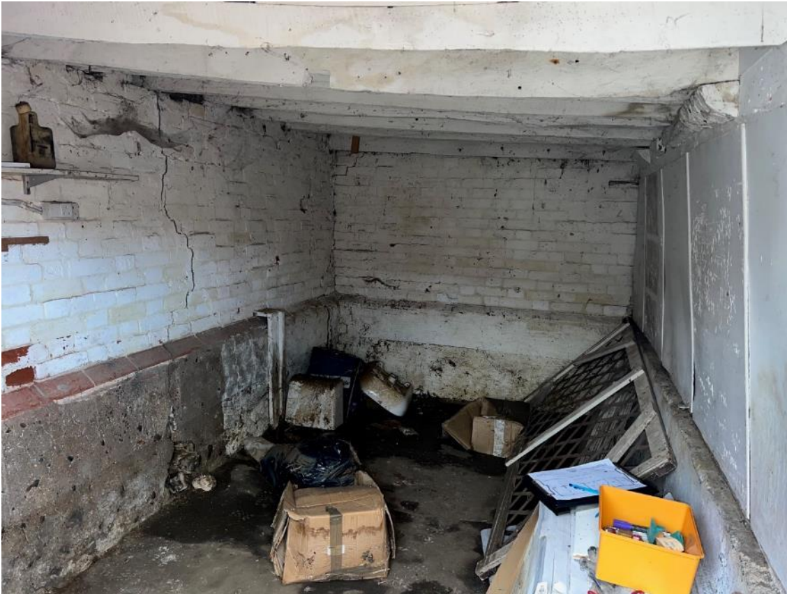
Photo 13. Internal view of The Barn, section B1. Shows vertical crack in southern wall to left.
