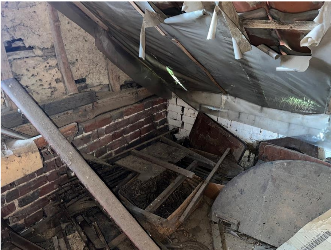
Photo 37. Shows south-west corner of loft space. Shows crack in wall. Gap between horizontal timber and brick work and light ingress.
