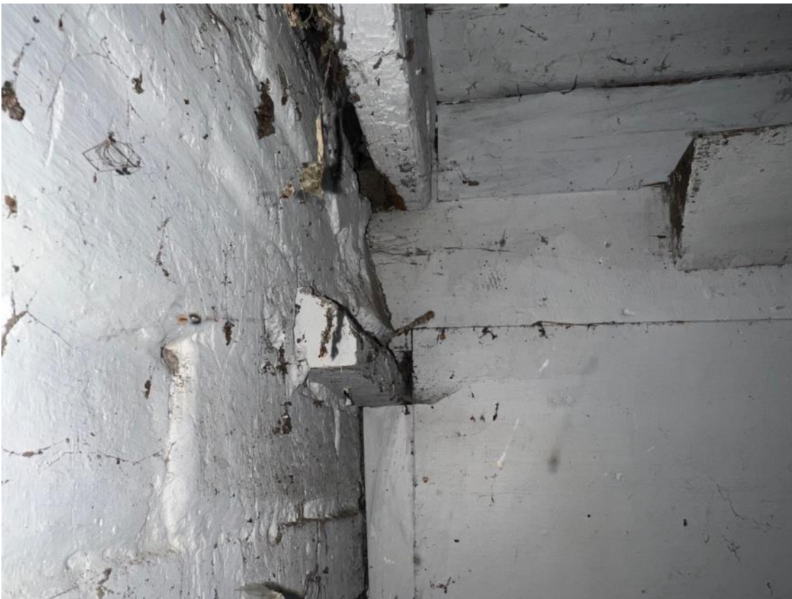
Photo 14. Shows gaps between timber and brickwork. B1.
