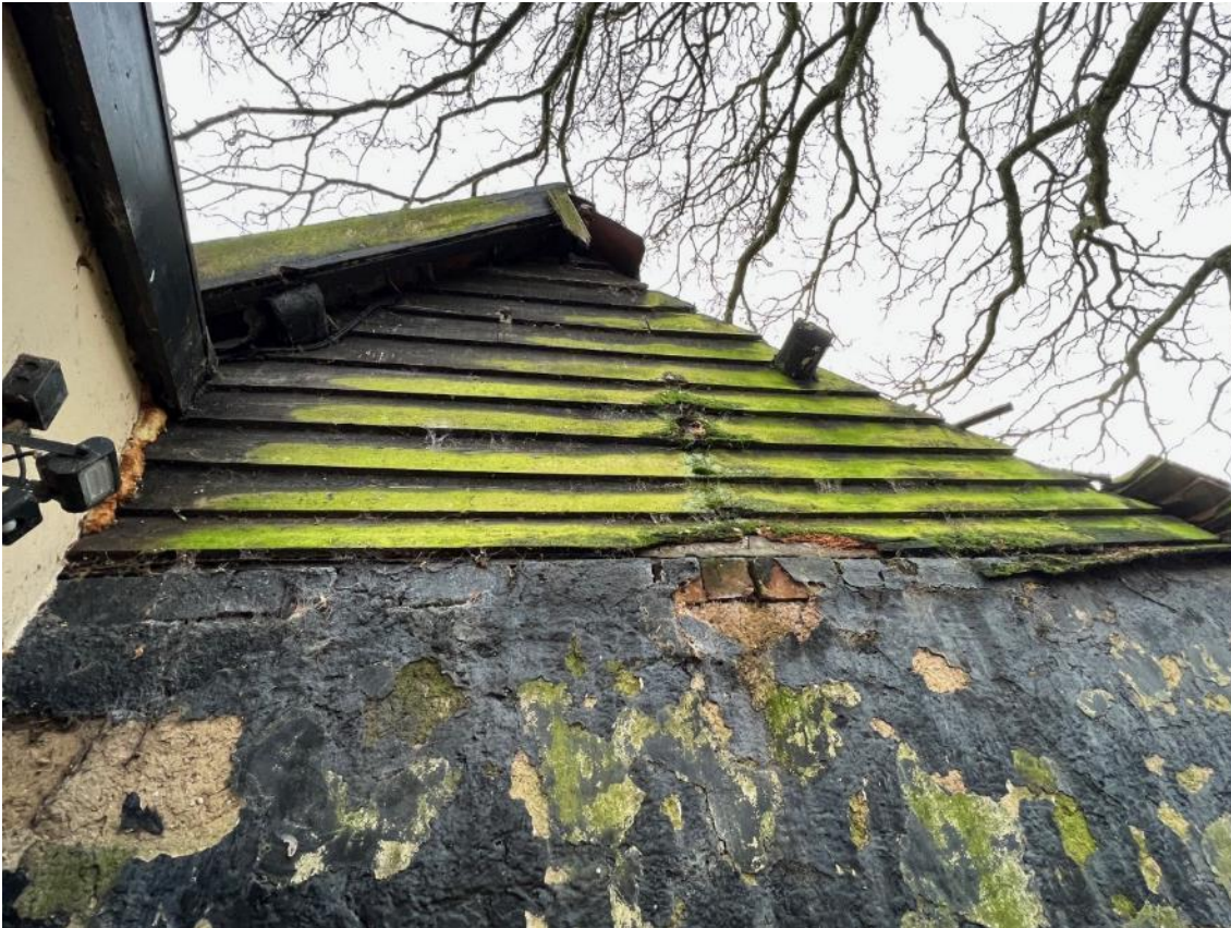
Photo 34. View of north gable end of the barn. Shows damaged brick work, missing soffit/fascia and lifted timber cladding.
