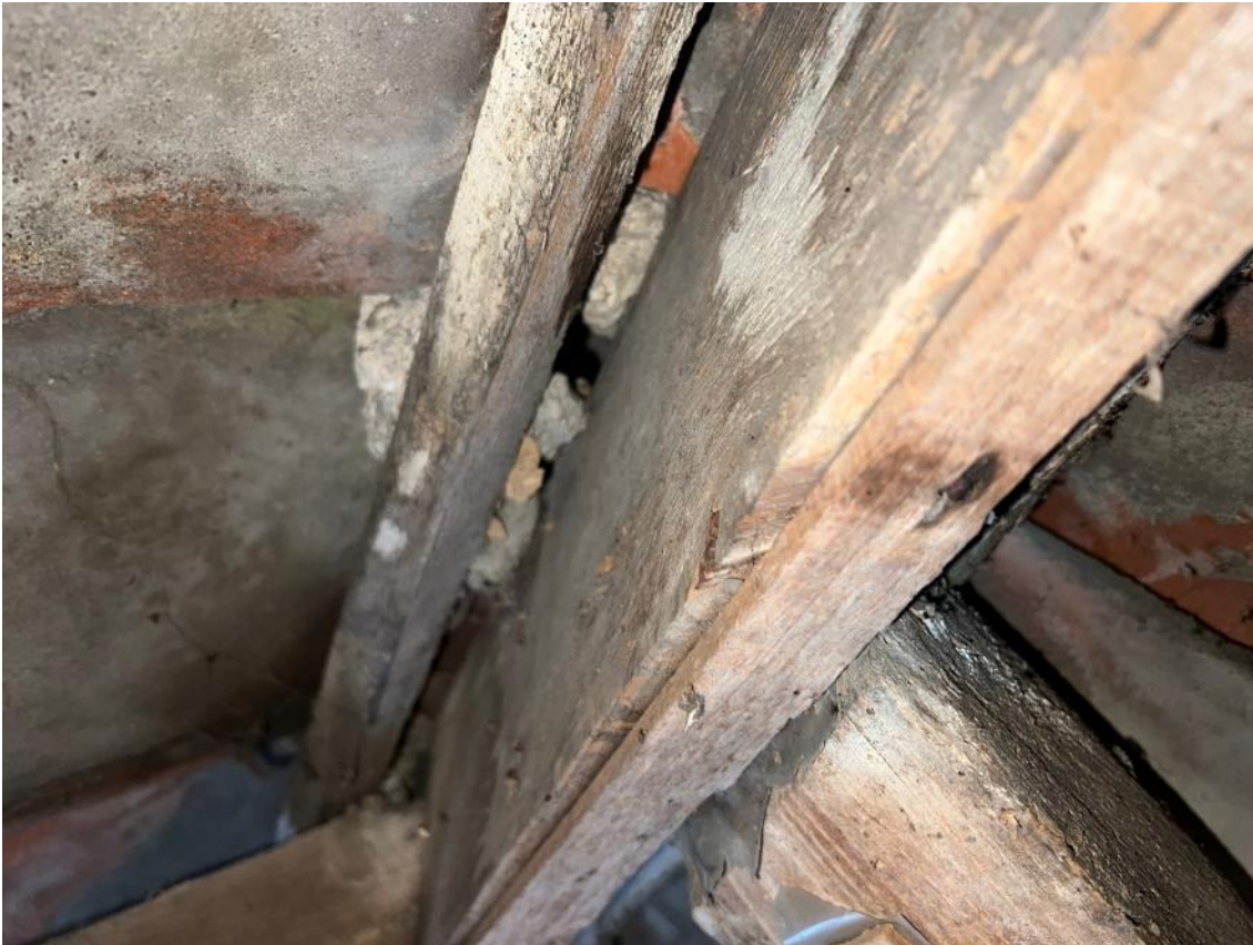
Photo 40. Shows gap between ridge board and purlins.
