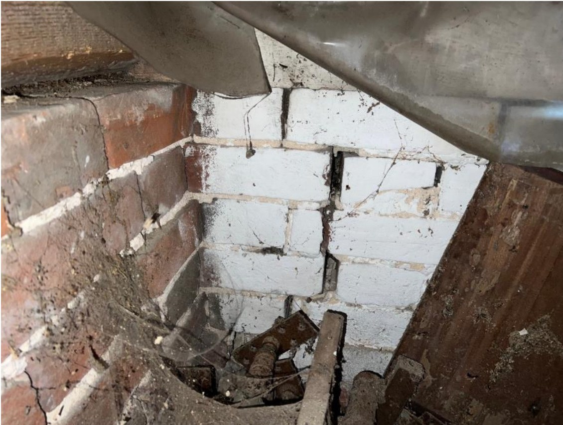
Photo 38. Shows close up of crack in brickwork shown in photo 27. Mostly filled with cobwebs.
