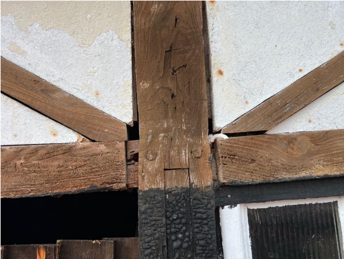
Photo 22. Exposed mortice and tenon joint and gaps between timber work. Located between B3 & B4.
