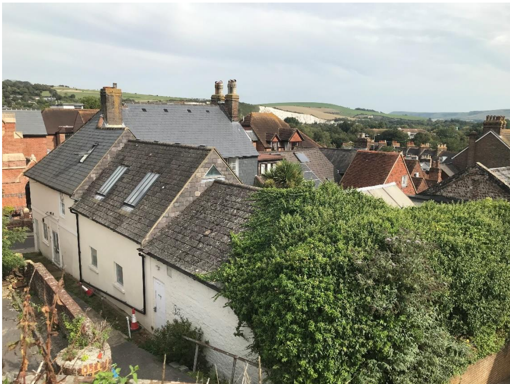
Figure 27: View southwest from the conservatory Terrace of the White Hart Hotel showing the prominence of the poor-quality fibre cement tile roof covering.
