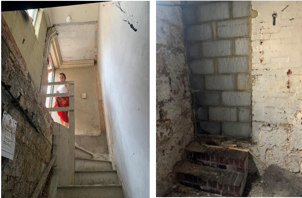
Figure 19: Basement stair of mid-20 th century date (left), the basement was originally accessed from No. 26 (right).
