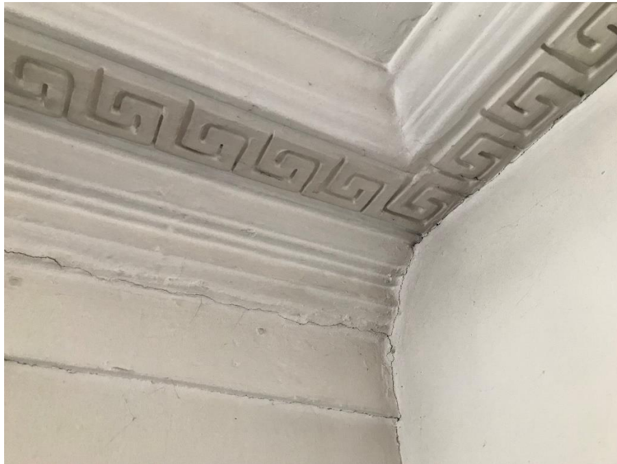
Figure 8: Truncated mouldings to the ground floor front room suggest possible communication with the stair hall in No. 26
