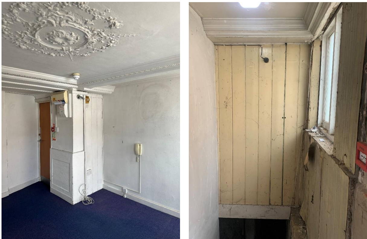
Figure 20: View of ground floor front room with mid 20 th century partition to right, inserted to form the basement stair (right) the upper part of which retains the original cornicing of the ground floor room
