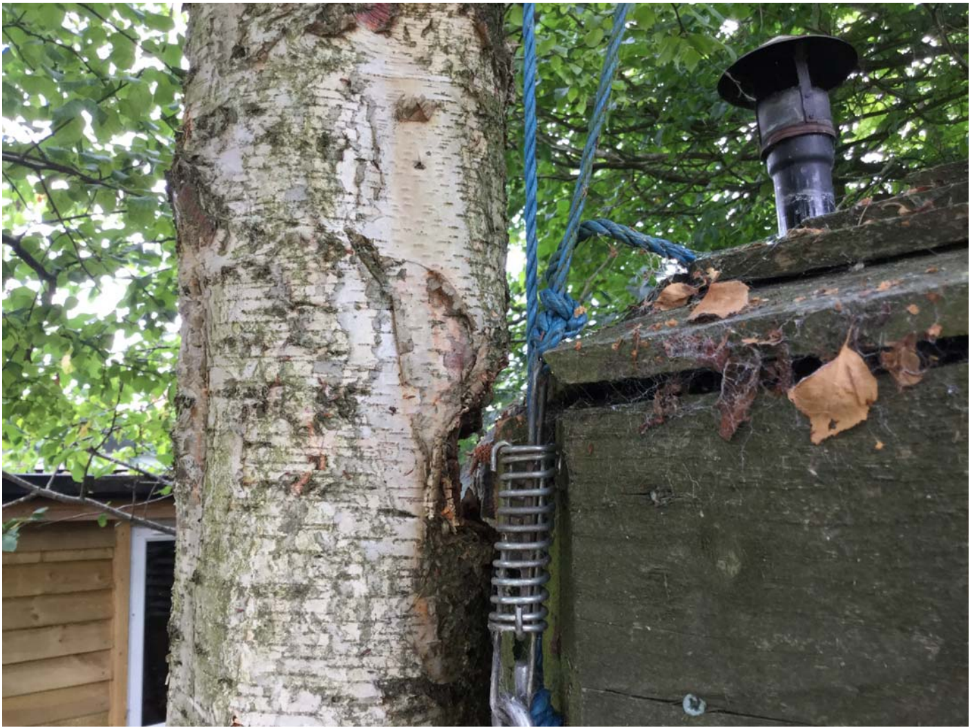
SAL3 T5 Birch rubbing against the adjacent structure.
