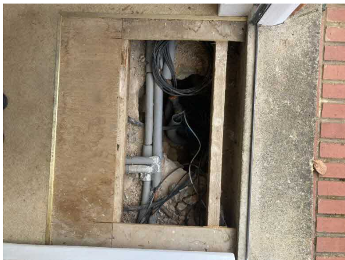
Fig. 7 Photograph of floor next to entrance door to 16 Albury Park Mews
