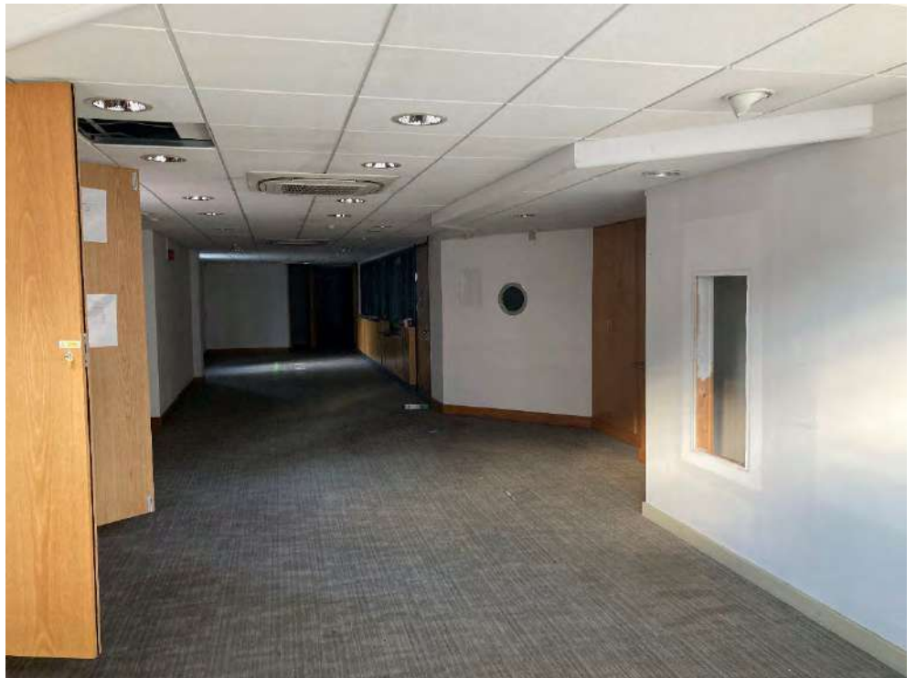
Plate 5 View north-west on the ground floor of 89 High Street illustrating the lack of remaining historic fabric.
