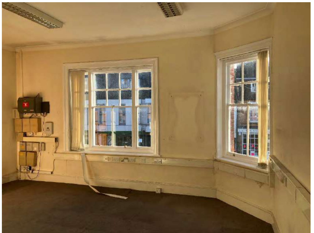
Plate 6 View south-east on the first floor of 89 High Street illustrating the lack of remaining historic fabric.
