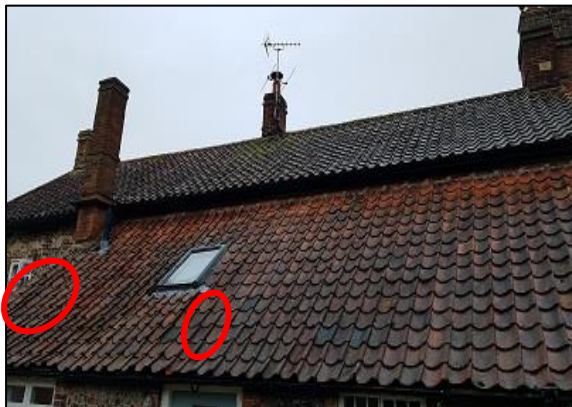
Figure 5: Western extension roof - lifted tiles circled.
