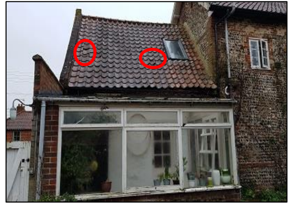
Figure 4: Northern wing – western aspect - lifted tiles circled.
