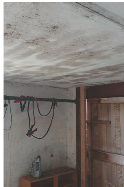
Damp and mould
