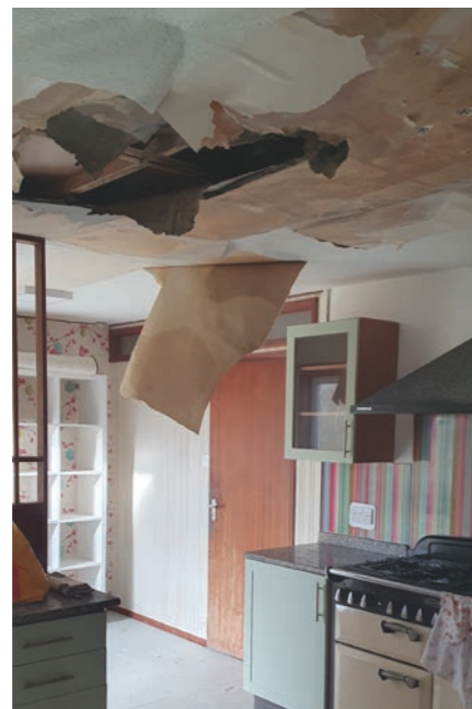
Broken pipework and damp
