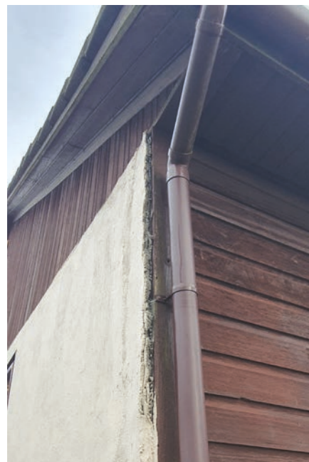
Failing render due to exposure
