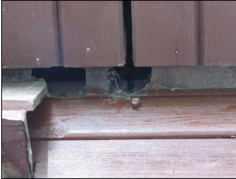
Figure 13. Damaged mesh has created a point of access on the western elevation.
