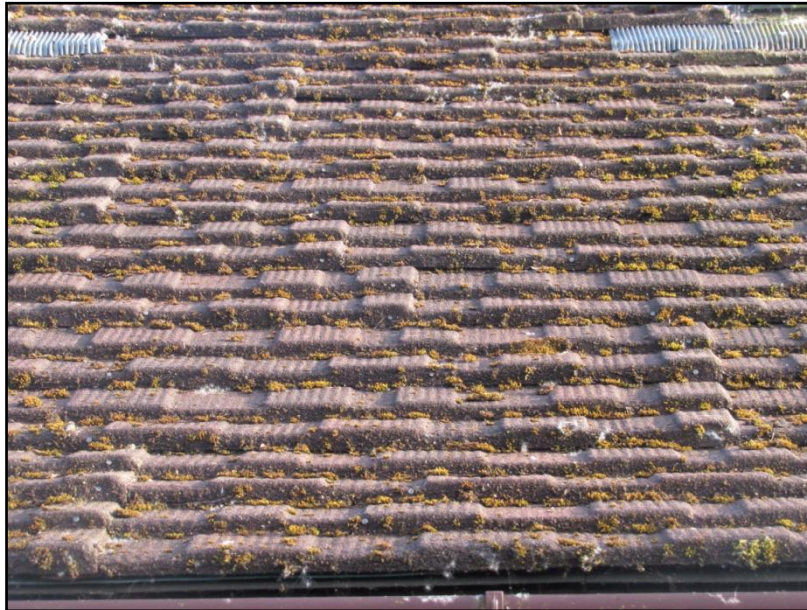
Figure 11. The roofing tiles create a continuous layer with no points of access.
