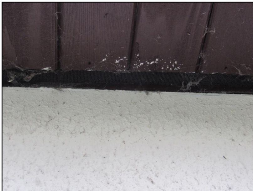
Figure 10. The building is tightly sealed around the eaves leaving no access to the wallhead.
