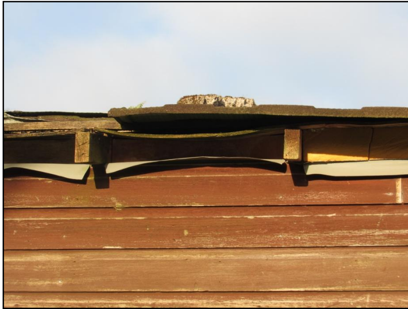
Figure 19. The Shed is open around the eaves.
