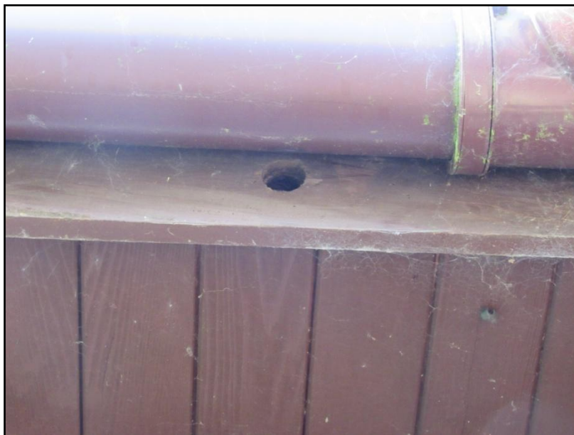
Figure 12. Small gap in the eaves on the western elevation.
