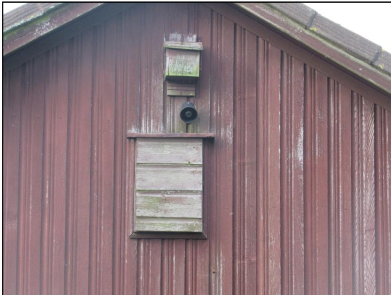
Figure 14. Large wooden vent with a bat box installed above on the southern elevation. The bat box was badly rotted and empty and the vent was filled with a large wasps nest – shown in Figure 15.
