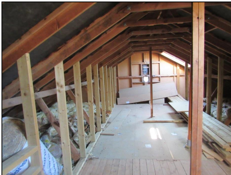
Figure 16. The roof void is timber framed and lined with a permeable fabric. There was no evidence of bat or birds in the building interior.
