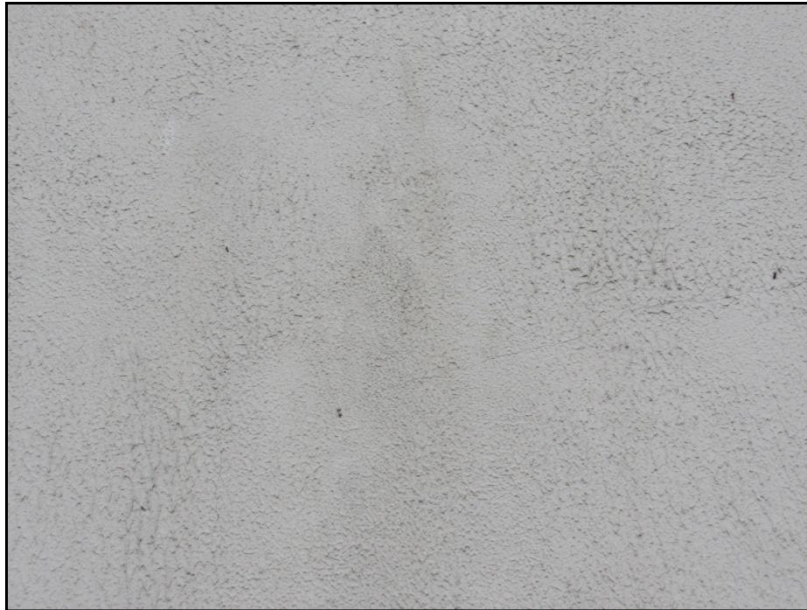
Figure 9. The external render is tightly sealed leaving no points of access.
