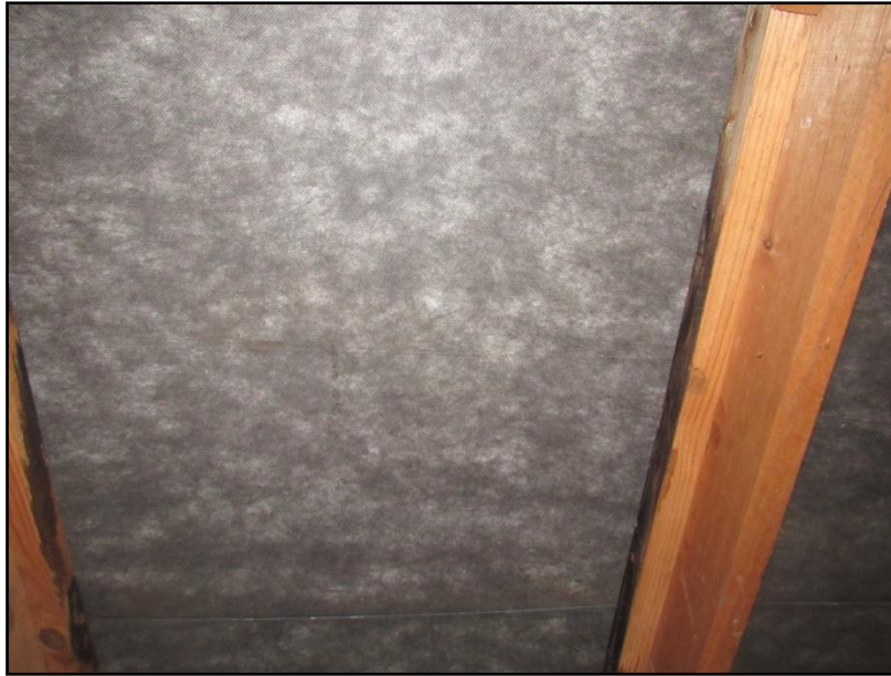
Figure 17. There is no sarking present within the roof void. The underside of the tiles is simply lined with a permeable fabric.
