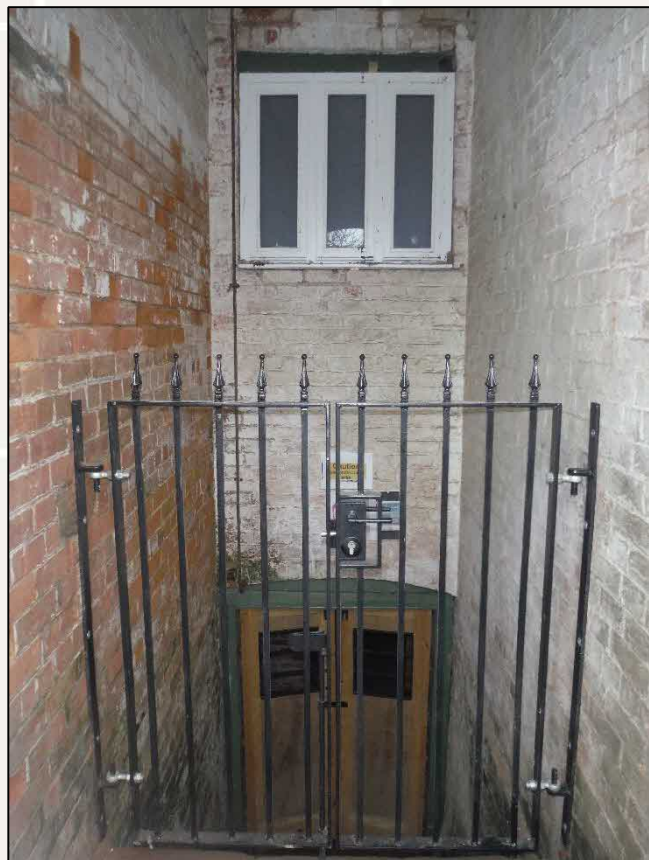
Image 2: Retained and enhanced (2no Kent bat box, baffles, cooling tower, locked barred door & gate, enhanced second access point) lesser horseshoe & brown long-eared hibernation and day roost in basement of Building 3.
