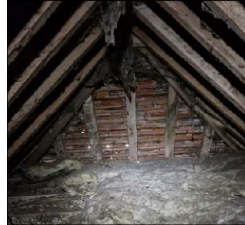
Image 18. View of void heading south over the original section of the building where bat droppings were located.
