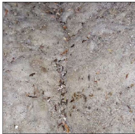
Image 21. View of cluster of bat droppings location in the centre of the void running north-south.
