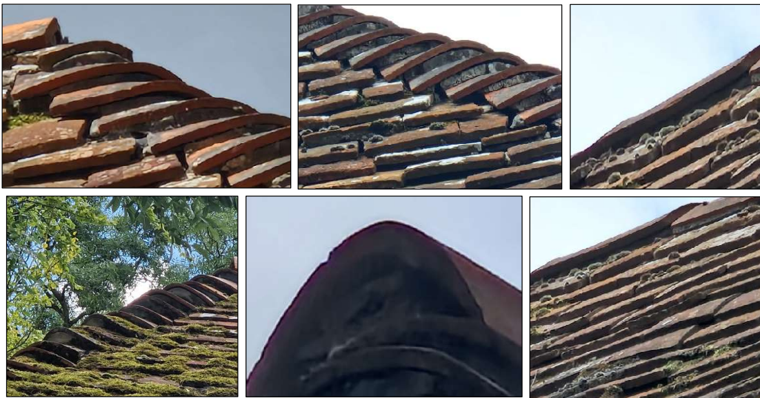
Image 11. Selection of potential roost features to the front and north facing roof hips within missing mortar, ridge tile gaps and lifted tiles.
