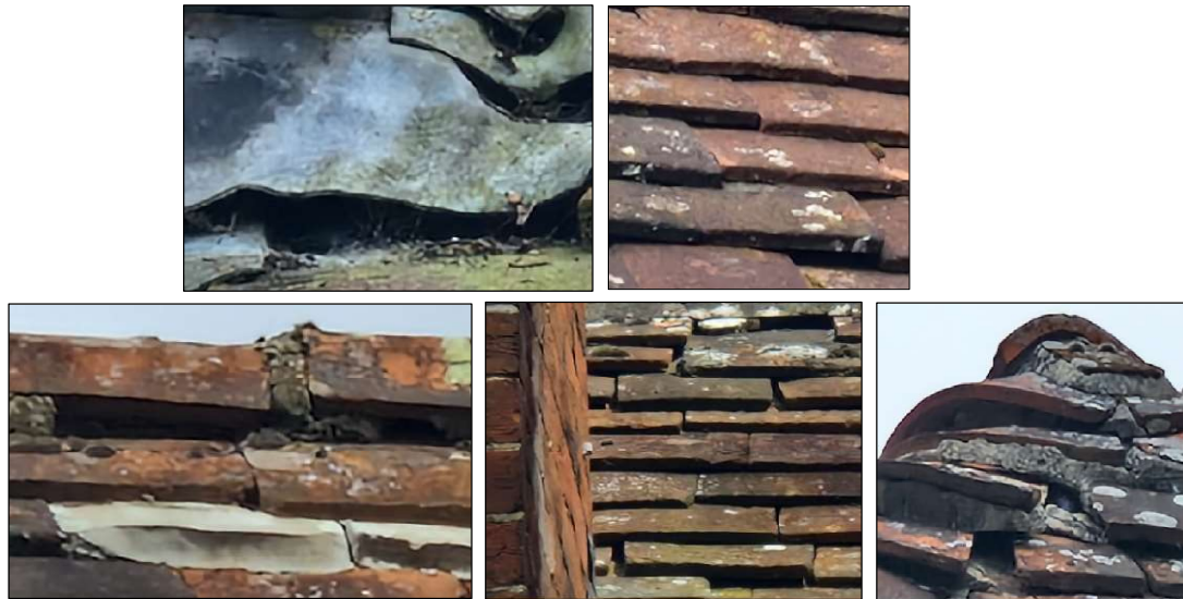
Image 12. Selection of photographs showing potential roost features in lifted roof tiles and flashing on the rear elevation.
