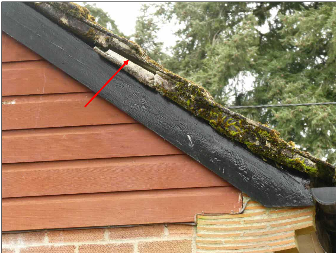
Figure 9. Missing mortar in verges. Southernwood, Woolton Hill. 21.03.23
