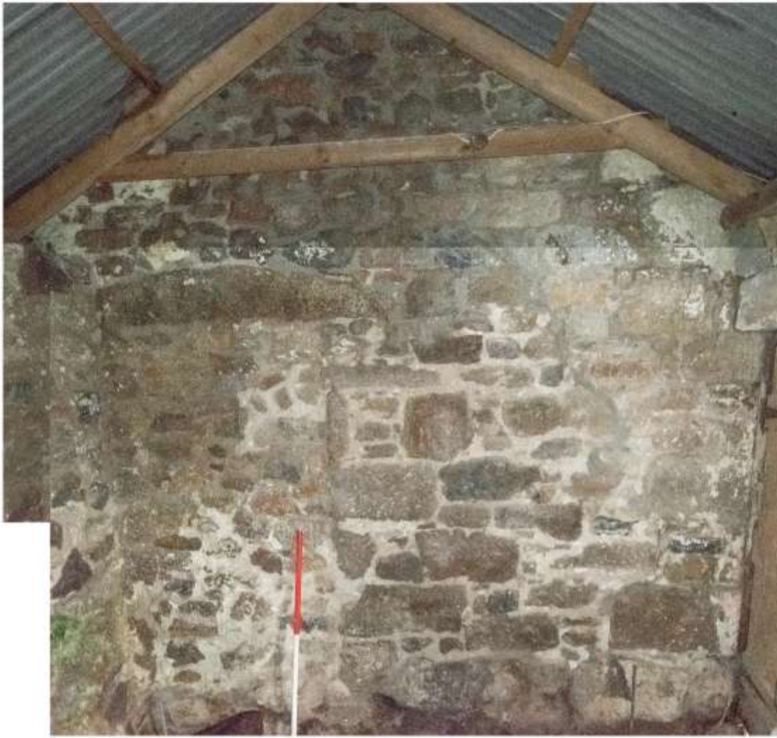
iii) Looking northwest, showing blocked door to B1a Composite image Archive refs: CHENH1223_0073.JPG; CHENH1223_0074.JPG Scale 1m
