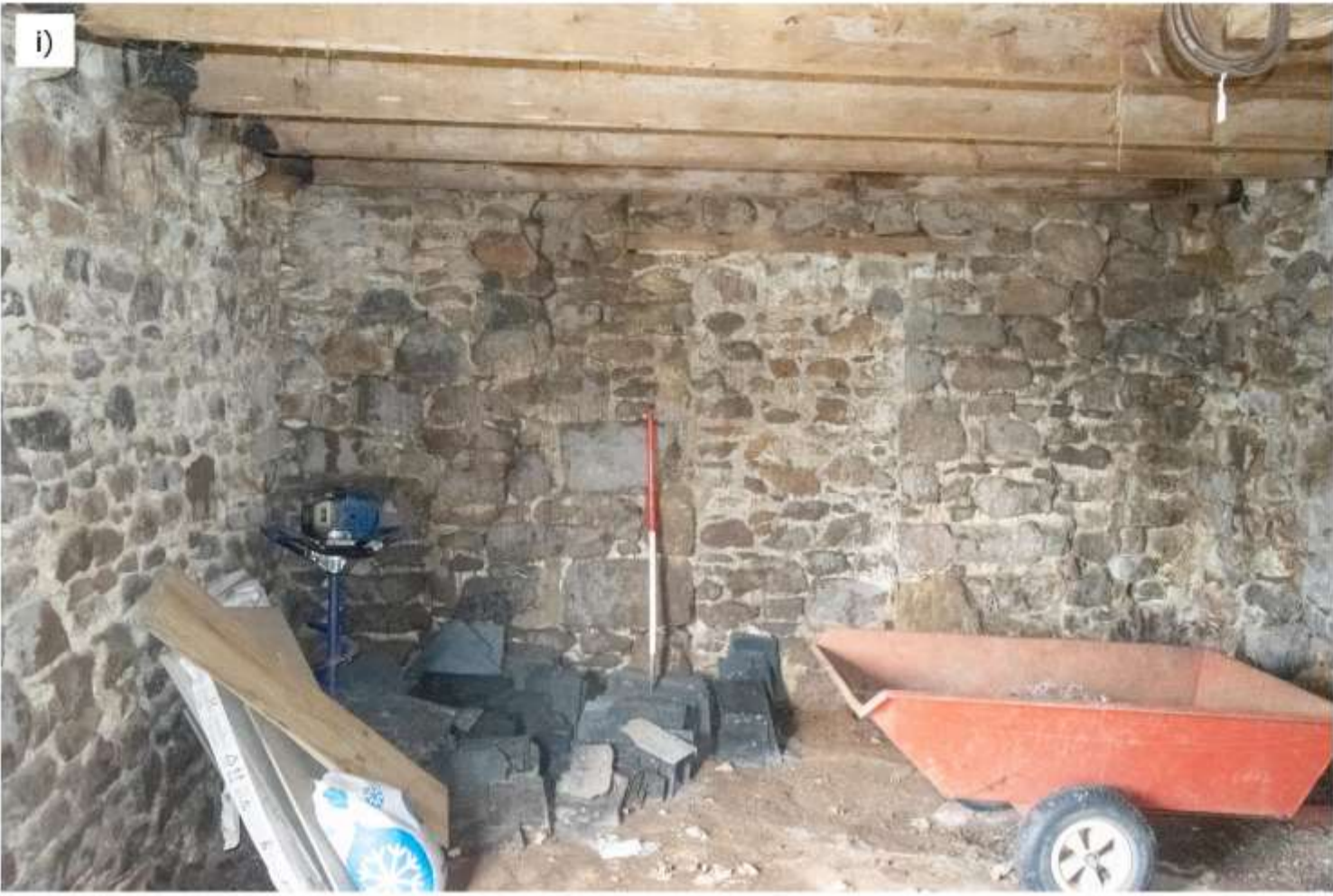
i) Looking southeast across the southern space beneath the granary. Note former doorway to Building 1C, blocked in granite rubble and lime mortar under a timber lintel.
