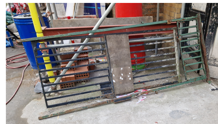
Existing gate, frame, and spandrel panel. Requiring various repairs.
