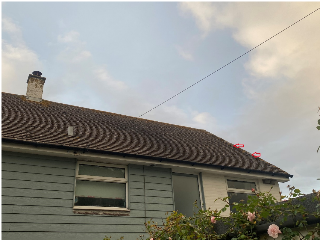
Figure 2. Southern elevation looking northeast. Red arrows showing potential access points for bats.
