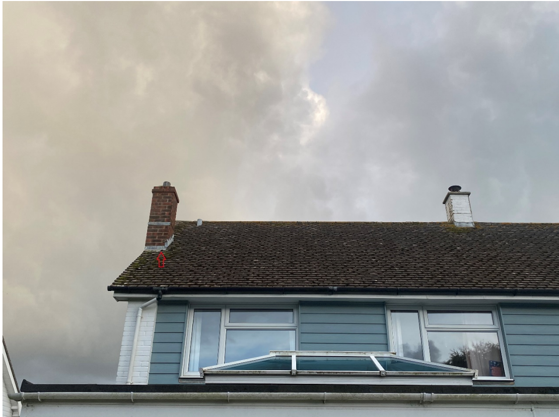
Figure 1. Northern elevations looking east. Red arrow showing potential access point for bats.
