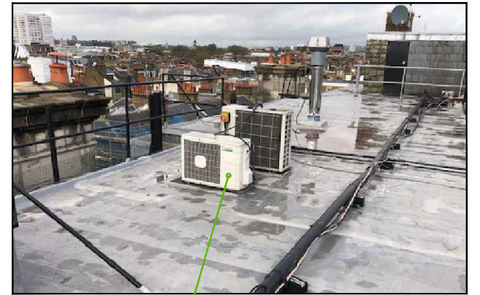
EXISTING AIR SOURCE HEAT PUMP UNITS (OTHER FLATS)
