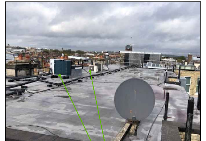
EXISTING AIR SOURCE HEAT PUMP UNITS (OTHER FLATS)
