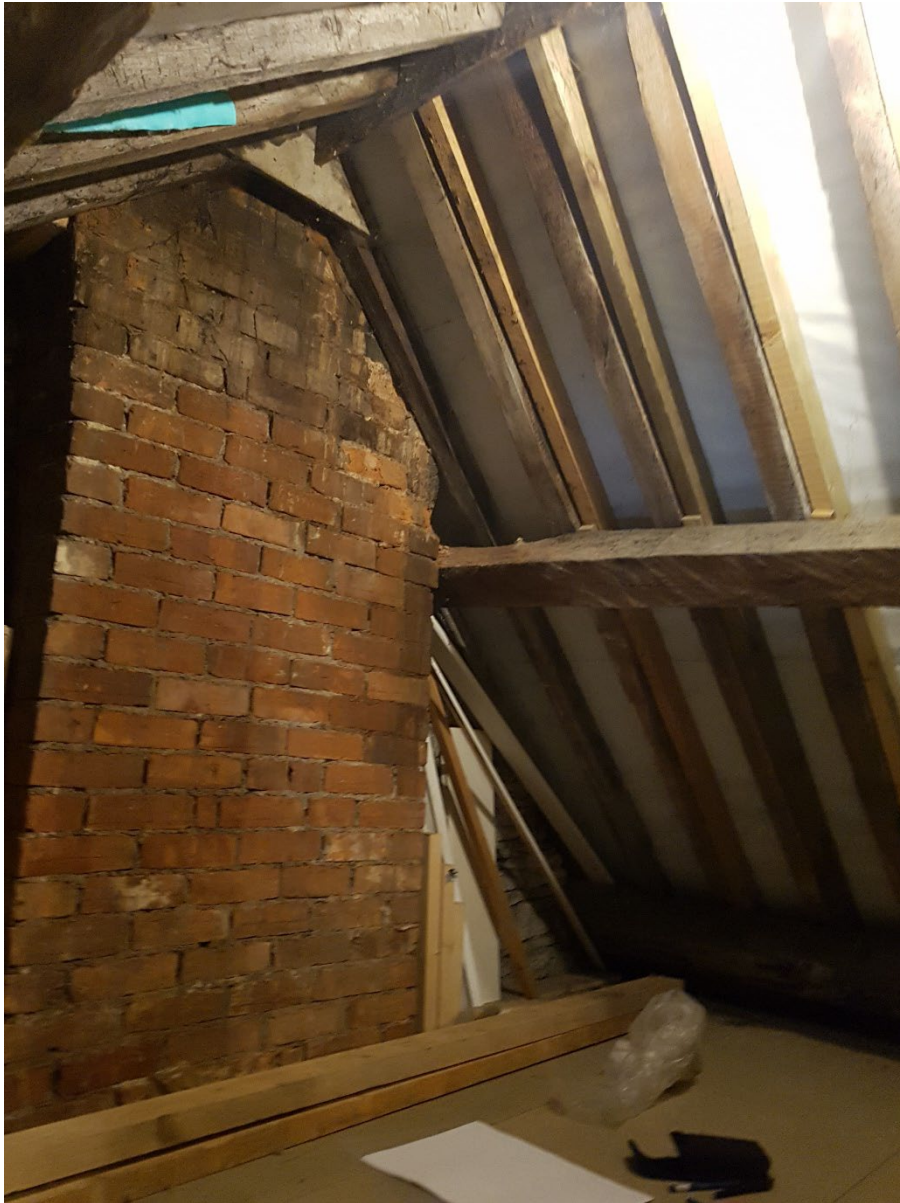
Attic – brick chimney breast and the roof slope to the street elevation showing modern breather membrane and rafters.
