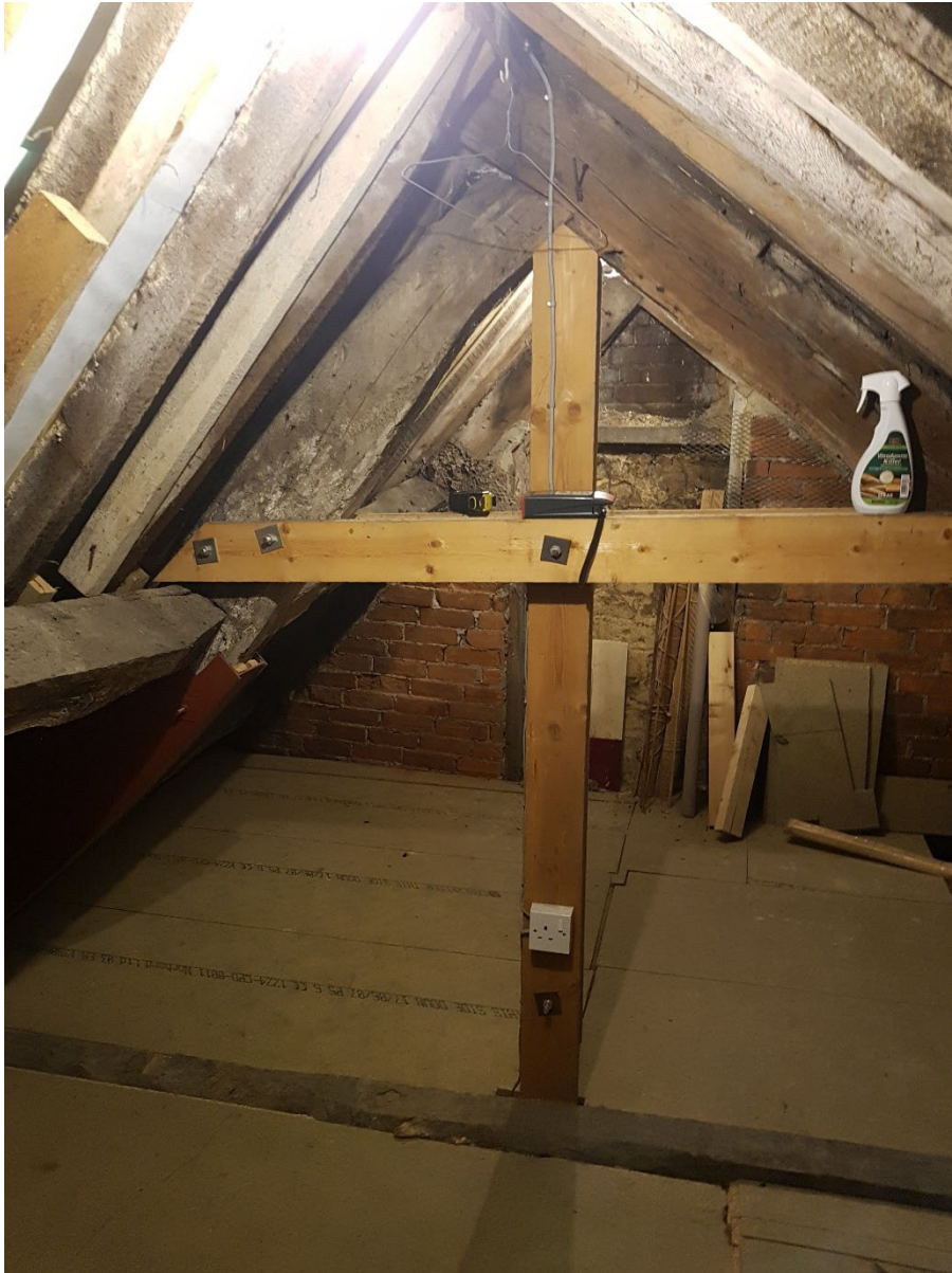
Attic – the bottom chord of the historic truss is visible in the floor. It appears that the ceiling below was raised up to line through with the truss and create storage space.
