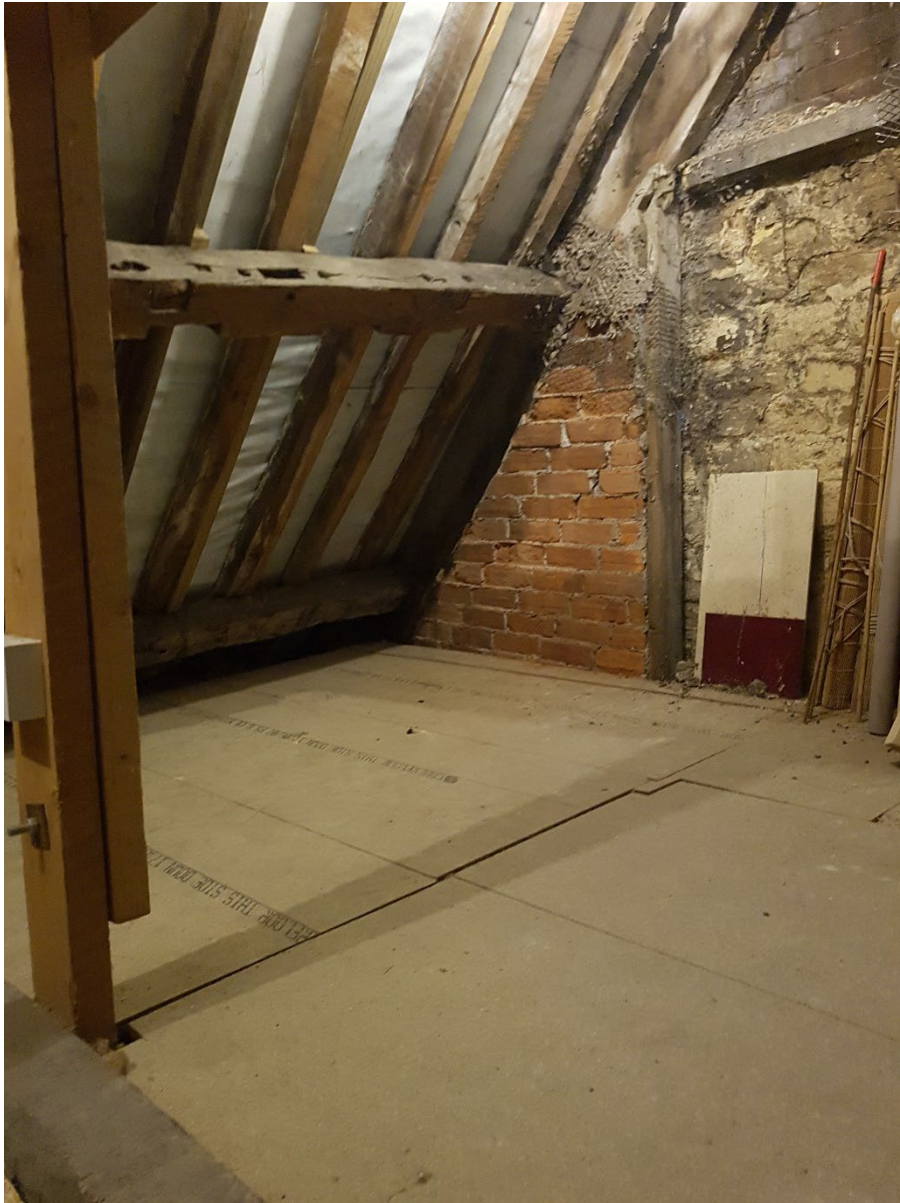
Attic – rafters are not contemporaneous with the purlins which may have been salvaged from another building given the notches which do not correlate with the rest of the roof structure.
