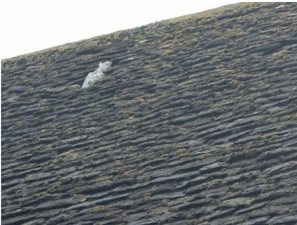
Photograph 5. Detail of roof tiles showing gaps under roof tiles.
