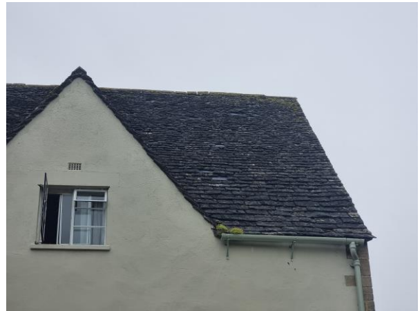
Photograph 4. Detail of the roof showing missing roof tiles.
