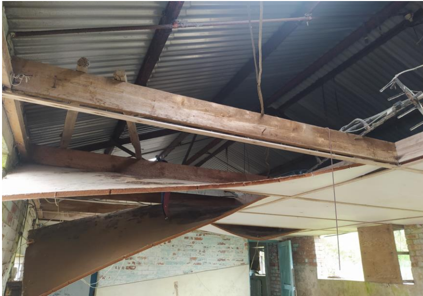
Figure 9 Partially boarded ceiling within Building 1; potential for nesting barn owl.
