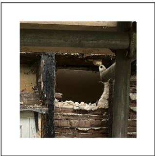
Visible damage to existing internal laths.
