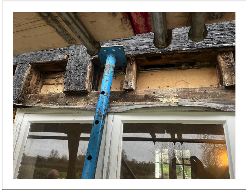
Structural timber in poor condition.
