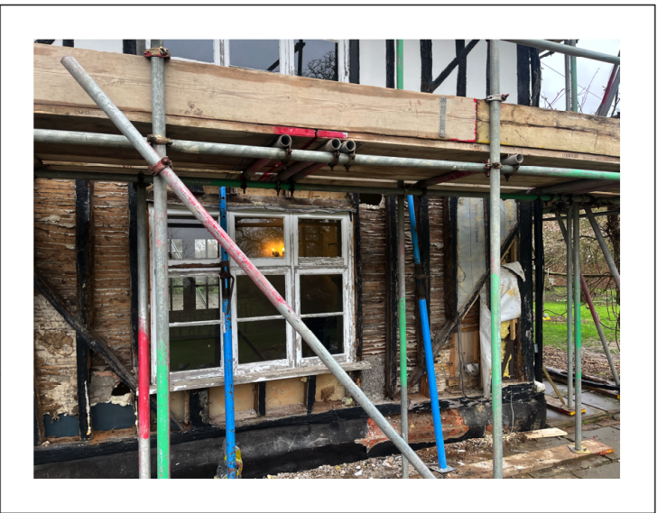
Inconsistent existing build up showing, timber laths, plaster board and galvanized metal laths within the historic timber frame.
