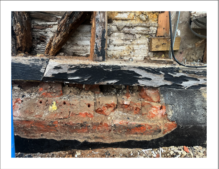
Brick plinth is currently in an extremely poor condition.
