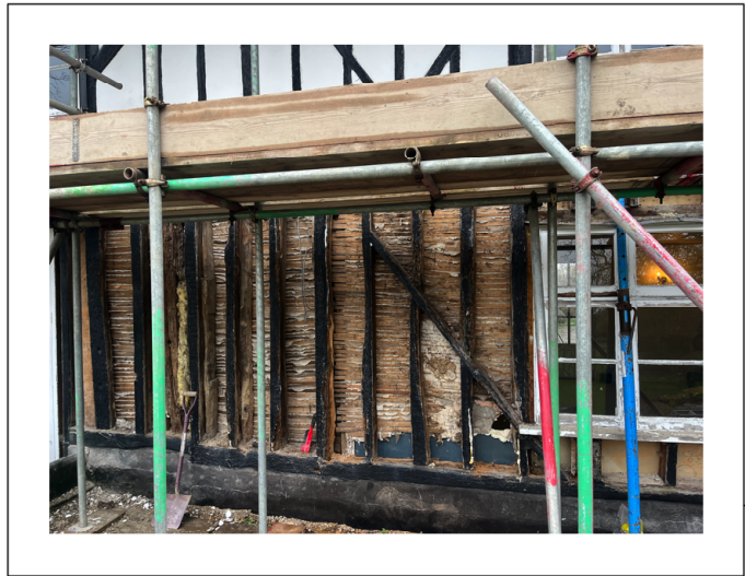
Visible damage to laths and plaster boarding.
