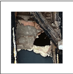
Visible damage to existing internal laths.
