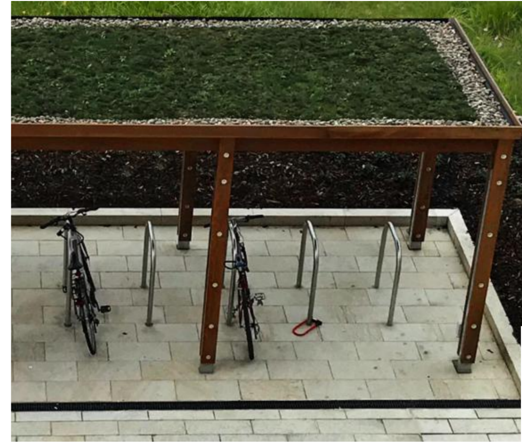
Cycle shelter- Indicative Image. Green roofing to cycle shelters as approved under Condition 17
