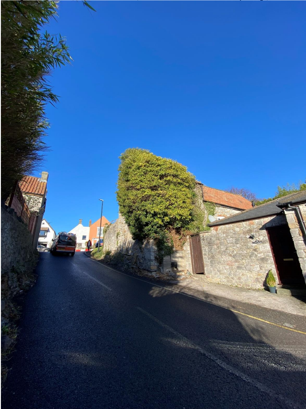
[View of outbuilding and overgrown, damaged / partially repaired masonry walls as viewed from The Scaurs]
