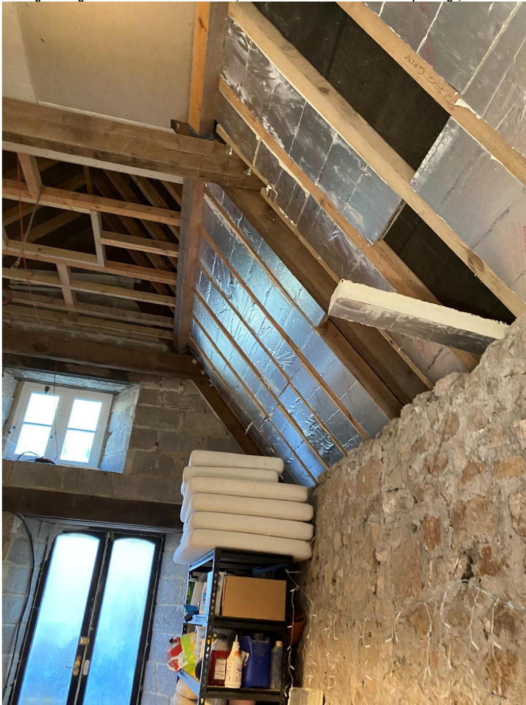
[Partially infilled rafters of repaired roof including ceiling at collar level. Stone and concrete blockwork walls on display]
