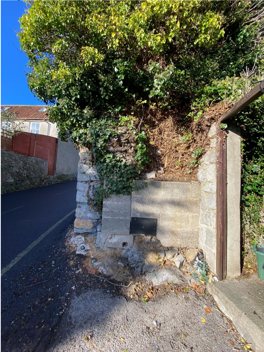
[View of outbuilding damaged / partially repaired masonry walls (to be repaired and restored as part of this proposal) as viewed from The Scaurs and off-road parking area]
