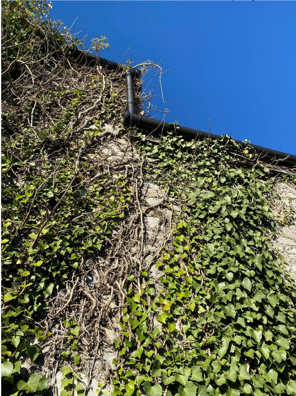
[Detached barn outbuilding remaining upvc rainwater goods and overgrown facades.]
