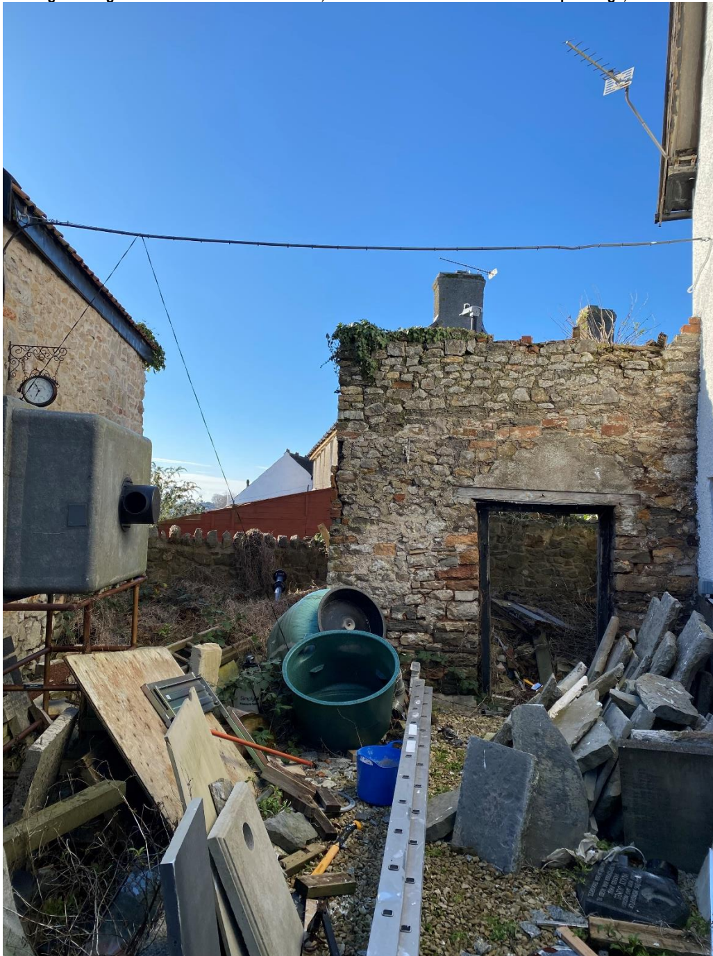
[dilapidated outbuilding and courtyard area, where it is proposed the extension is located]
