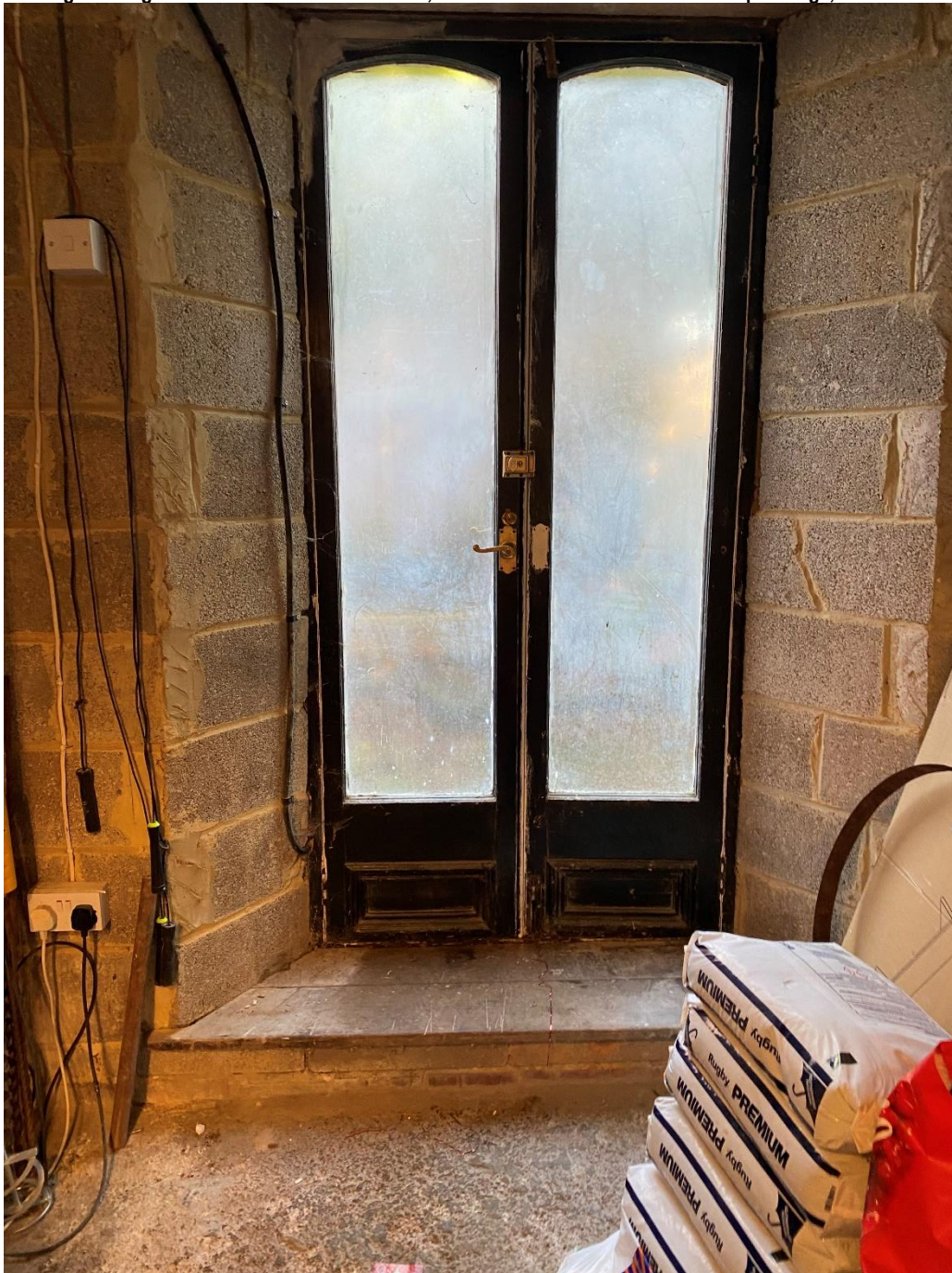
[detached barn entrance doors, step and concrete ramping]
