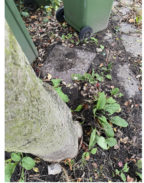
T1 - Holly root proximity to access chamber
