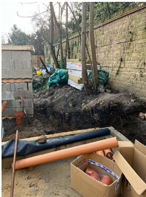
T4 & T5 - Sycamore unstable root area
