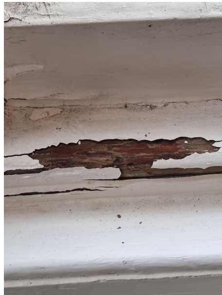
Rotting internal sills
