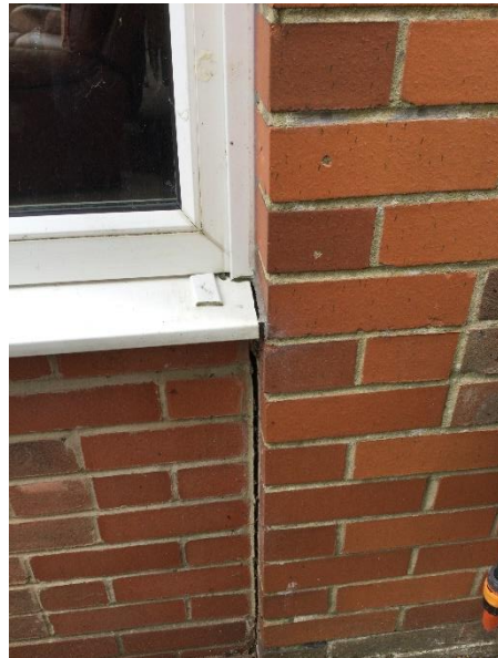
Gap at the junction of the left-hand wall and the main property
