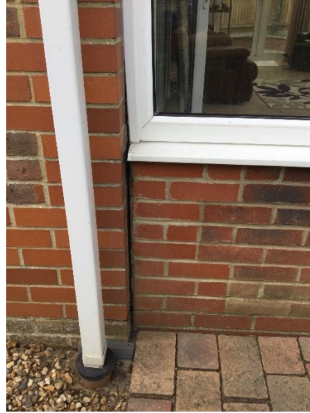
Gap at the junction of the right-hand wall and the main property
