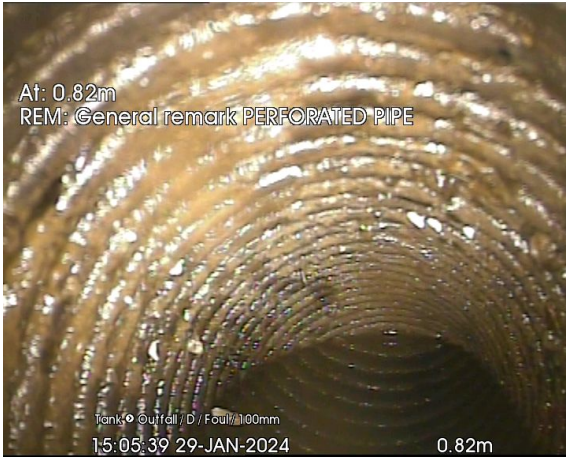
1_0-82m_150539.jpg, 00:00:20, 0.82 m General remark, PERFORATED PIPE
