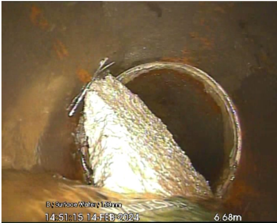
B:\Surface Water\133mm 14:51:15 14-FEB-2024 6.68m SWMH3X_97918841-b6ab-4752-98de-a92e181b85d6_20240 220_135933_332.jpg, 00:00:45, 6.68 m Other obstacles from 4 o'clock to 9 o'clock, 55% cross-sectional area loss, Believed to be lump of concrete
