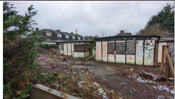
Photograph 6– Recently cleared small trees and shrubs that grew through the hardstanding layer.
