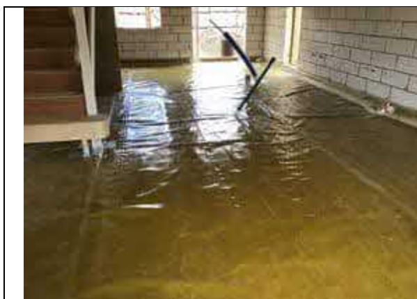
Plot 35 overview of installed Visqueen HC Blok Gas Barrier as an infill.
