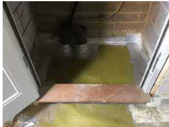
Sealed pipe penetrations in riser cupboard to apartment block c.
