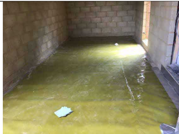
Overview of installed membrane to the garage, as an infill to plot 70.
