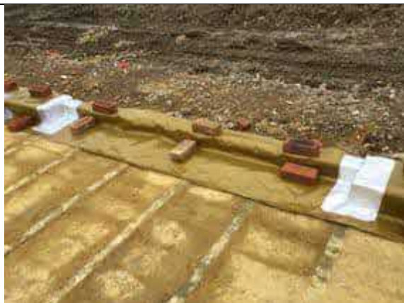
Plot 6 typical door threshold seal using SAGM.
