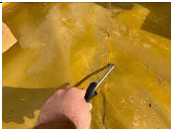
Plot 63 FOG Unit - Pick test upon a successfully hand welded lap joint.
