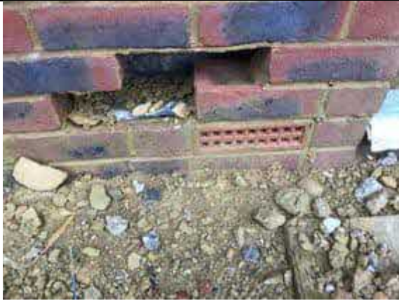
Air brick in place at the time of our inspection to plot 49.
