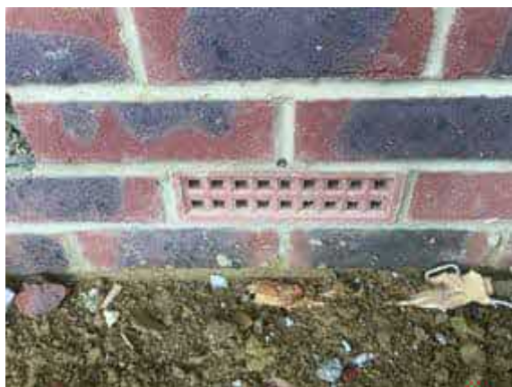
5no air bricks per plot were in place at the time of our inspection.
