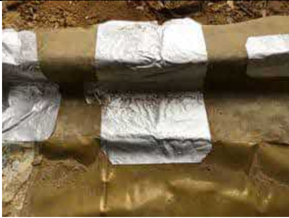
Plot 27 patch repair using SAGM to damage caused by follow on trades.
