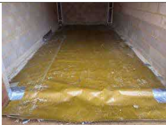
Overview of Visqueen HC Blok infill installation to Plot 30 FOG Unit Garage.
