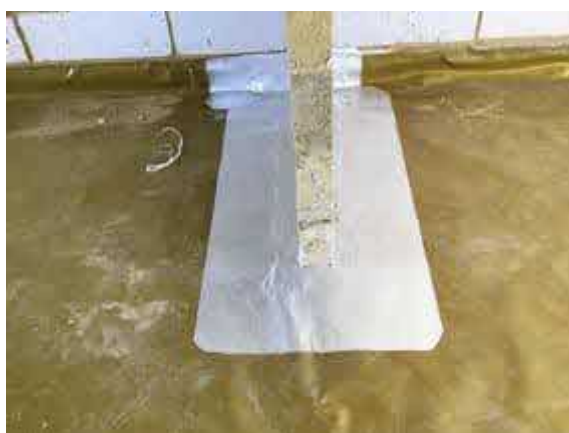
Plot 3 retro fit detail over the damaged membrane that is under the internal block work wall.
