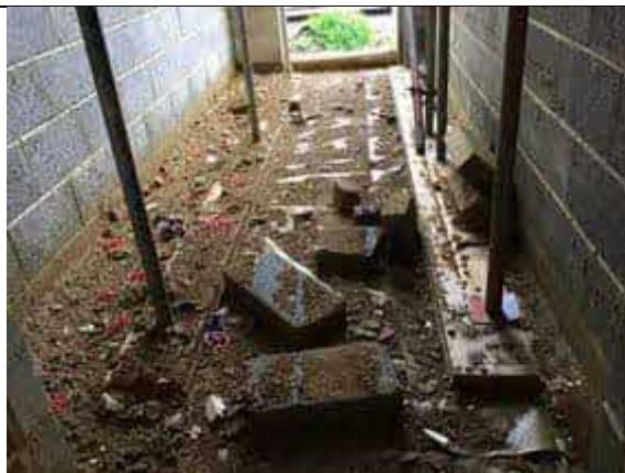
Incomplete cycle store.
