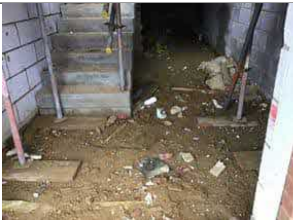
Incomplete stair lobby.
