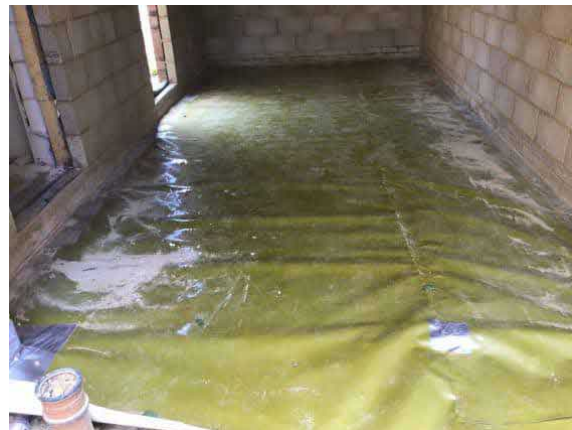
Overview of installed membrane to the garage, as an infill to plot 72.
