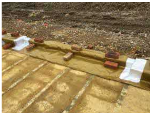
Plot 6 typical door threshold seal using SAGM.
