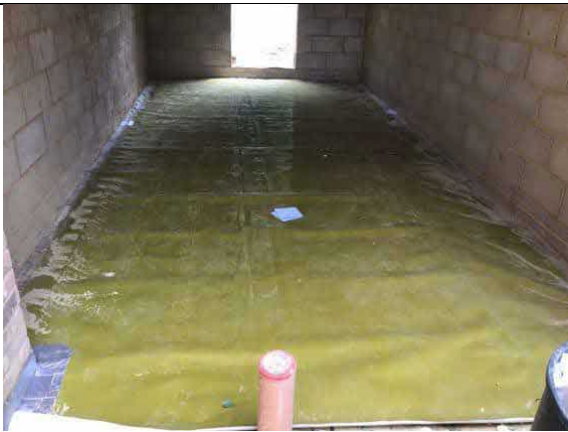
Overview of installed membrane to the garage, as an infill to plot 69.
