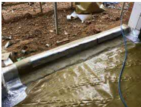
Repaired damaged to the door threshold due to follow on trades using SAGM.
