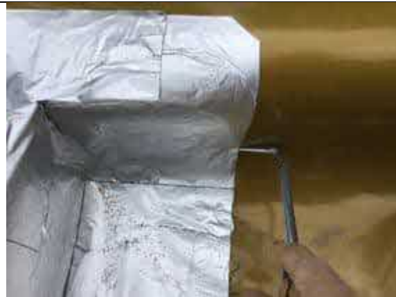
Plot 74 pick testing all SAGM detailing.
