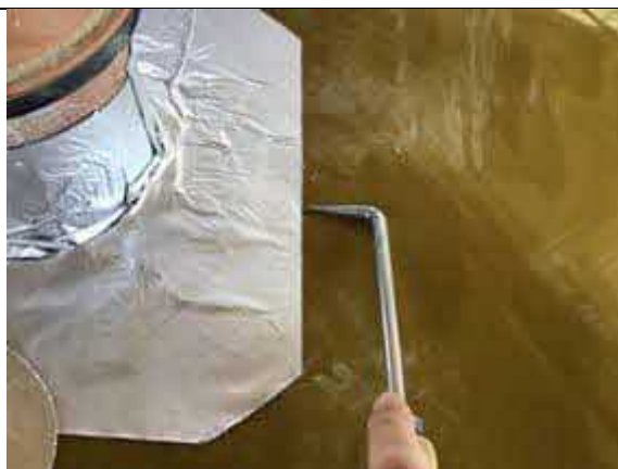
Plot 76 pick testing all SAGM detailing.
