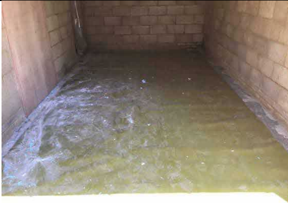
Overview of installed membrane to the garage, as an infill to plot 40.
