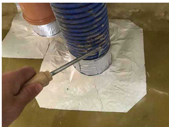
Pick testing all SAGM detailing in plot 52.
