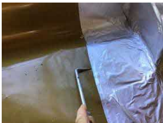
Plot 3 pick testing all SAGM detailing.
