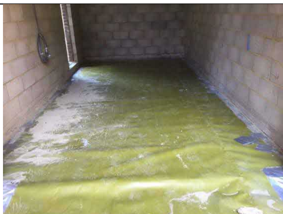
Overview of installed membrane to the garage, as an infill to plot 74.
