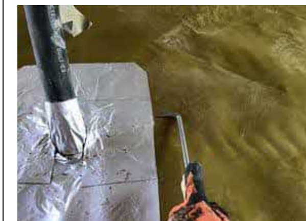
Plot 35 pick testing all SAGM detailing.
