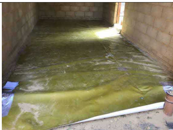
Overview of installed membrane to the garage, as an infill to plot 73.
