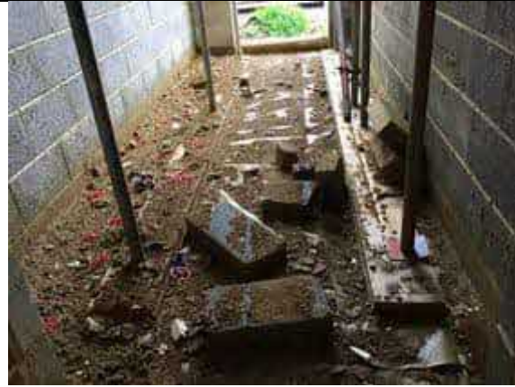
Incomplete cycle store.
