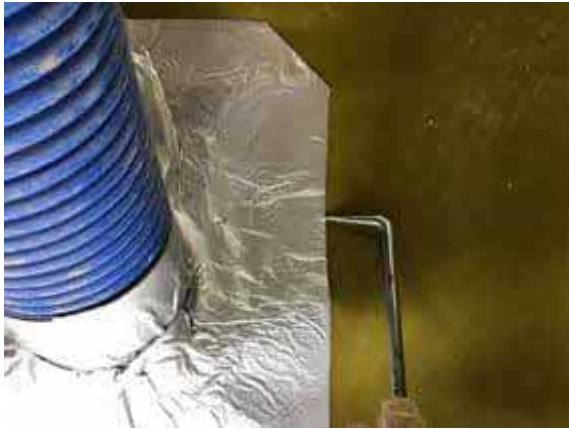
Pick testing all SAGM detailing in plot 50.
