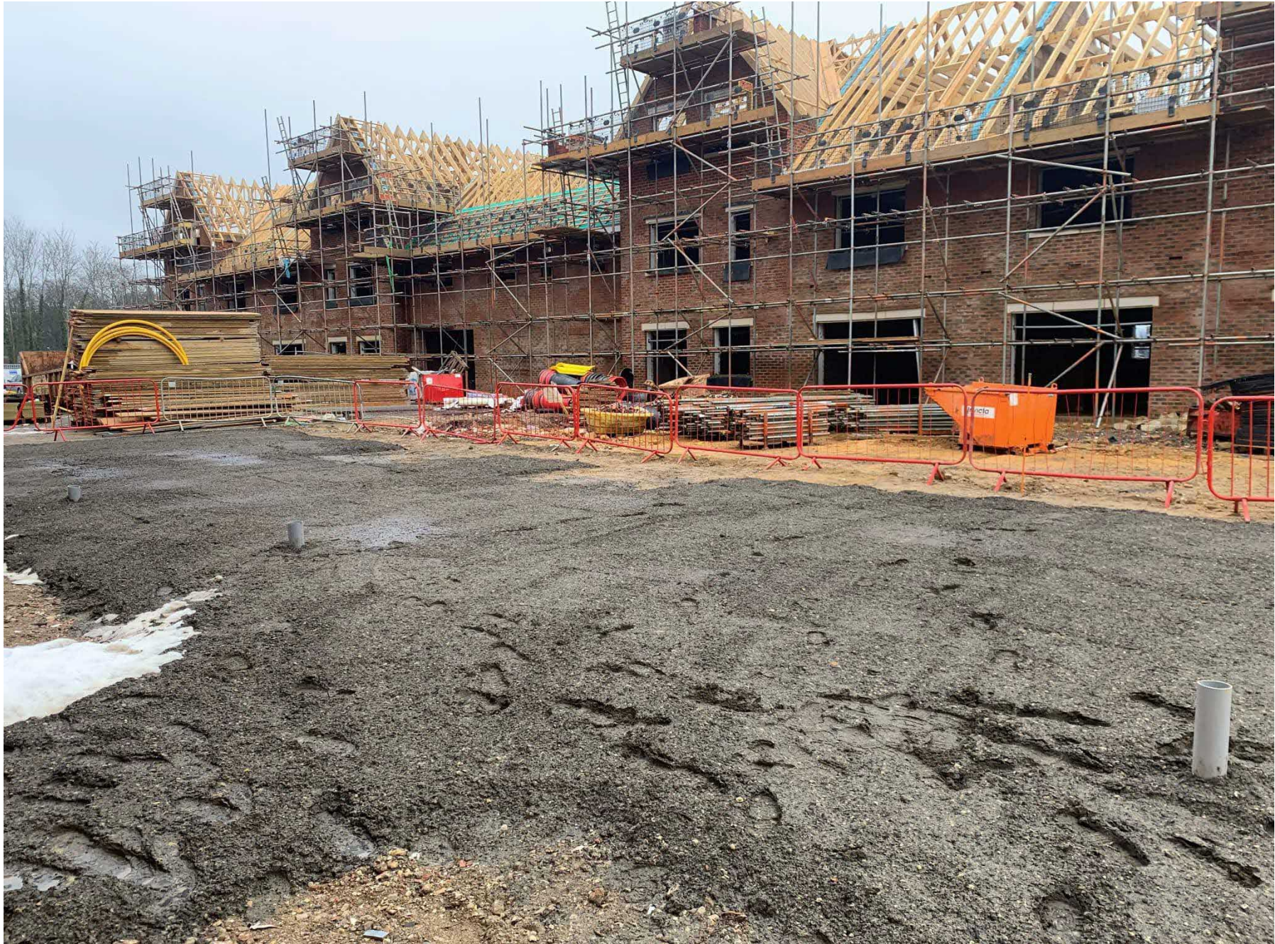
Photo 6: Plot 32-35 Rear Gardens showing the topsoil layer. Grey tubes reveal the subsoil and geotextile layers.
