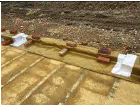
Plot 6 typical door threshold seal using SAGM.
