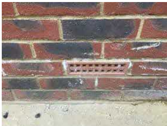
Air brick in place at the time of our inspection to plot 65.
