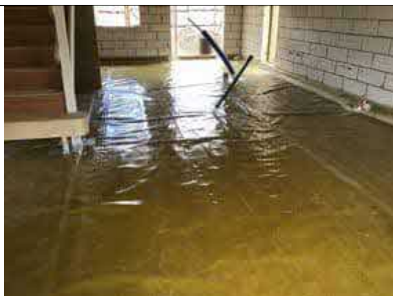
Plot 35 overview of installed Visqueen HC Blok Gas Barrier as an infill.
