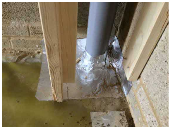
Sealed pipe penetration using SAGM to the rear of the garage plot 45.
