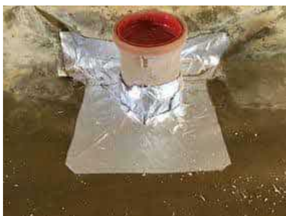
Typical pipe penetration seal using SAGM to plot 65.
