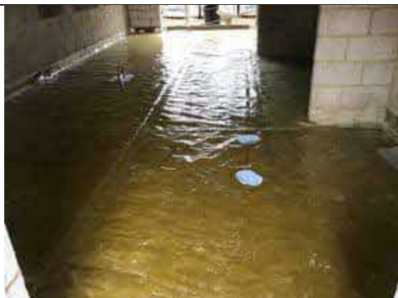
Plot 33 overview of installed Visqueen HC Blok Gas Barrier as an infill.
