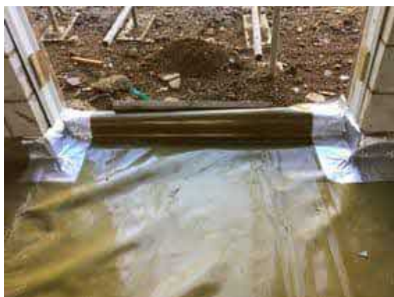
Plot 2 typical door threshold seal using SAGM.
