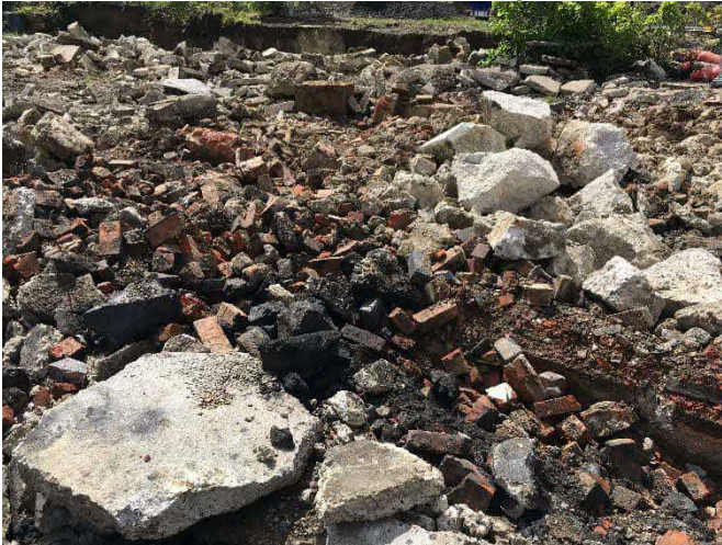
Broken out concrete in NE corner.
