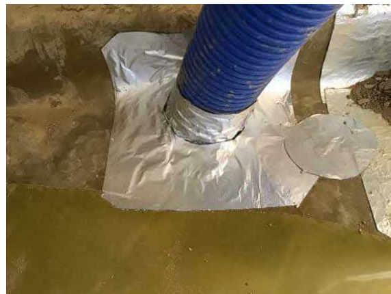
Typical pipe penetration seal using SAGM to plot 46.
