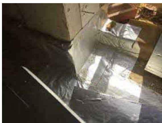
Re sealed door threshold detail using SAGM to plot 65.
