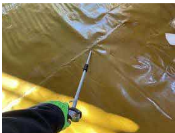
Plot 73. Air lance integrity test conducted upon all hand welded membrane lap joints.
