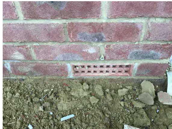
Air brick in place at the time of our inspection to plots 51-53.
