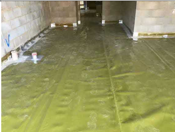
Overview of installed Visqueen HC Blok gas membrane, that has been installed as an infill to Apartment block H.
