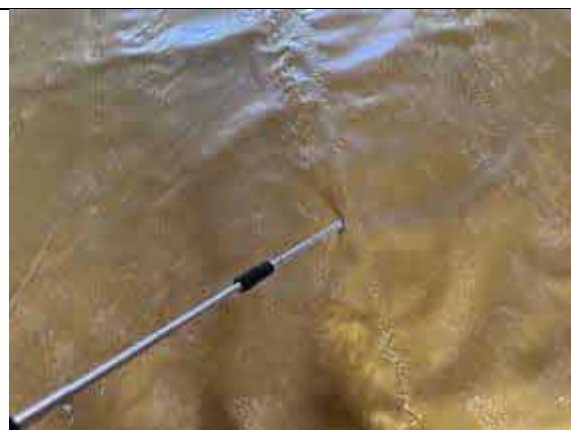
Plot 29 - Air lance integrity test upon a hand welded membrane lap joint.
