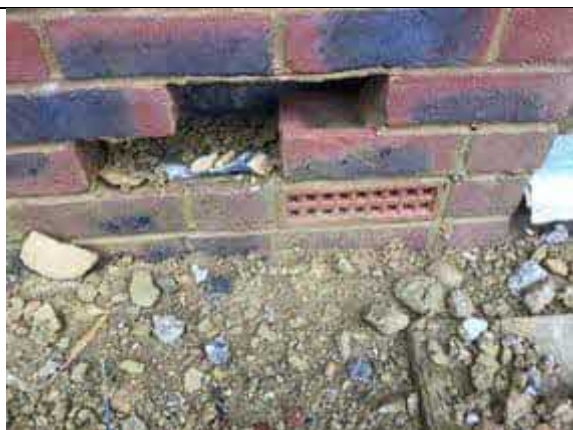
Air brick in place at the time of our inspection to plot 49.
