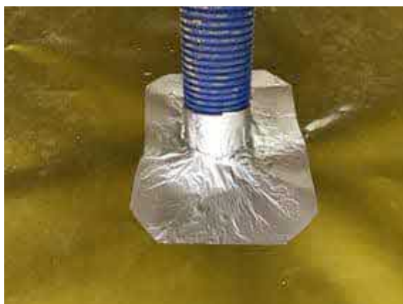
Typical pipe penetration seal using SAGM to plot 50.
