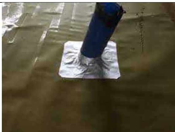
Typical pipe penetration seal using SAGM to plot 39.
